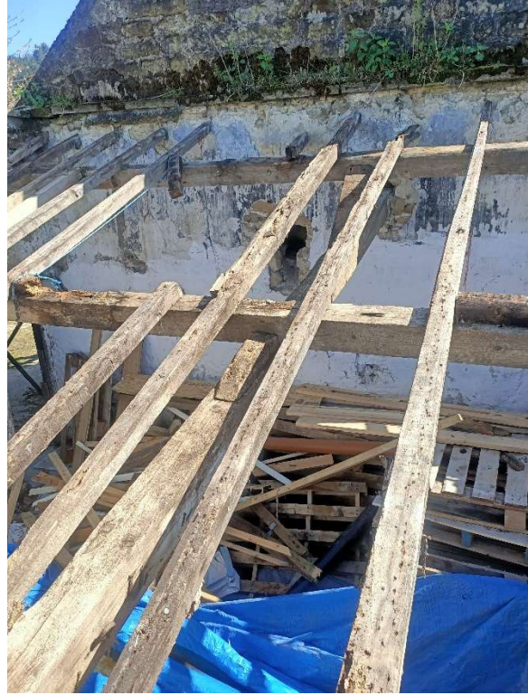
Vernacular alteration and general decay
