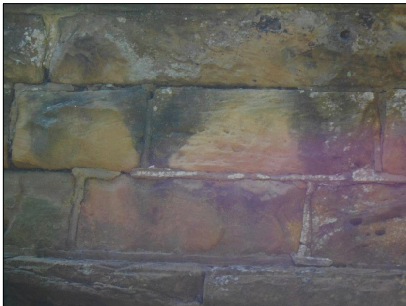
Figure 4: Minor crevices in east side
