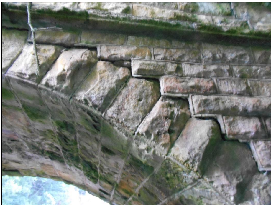
Figure 8: Substantial crack at south-west corner of bridge
