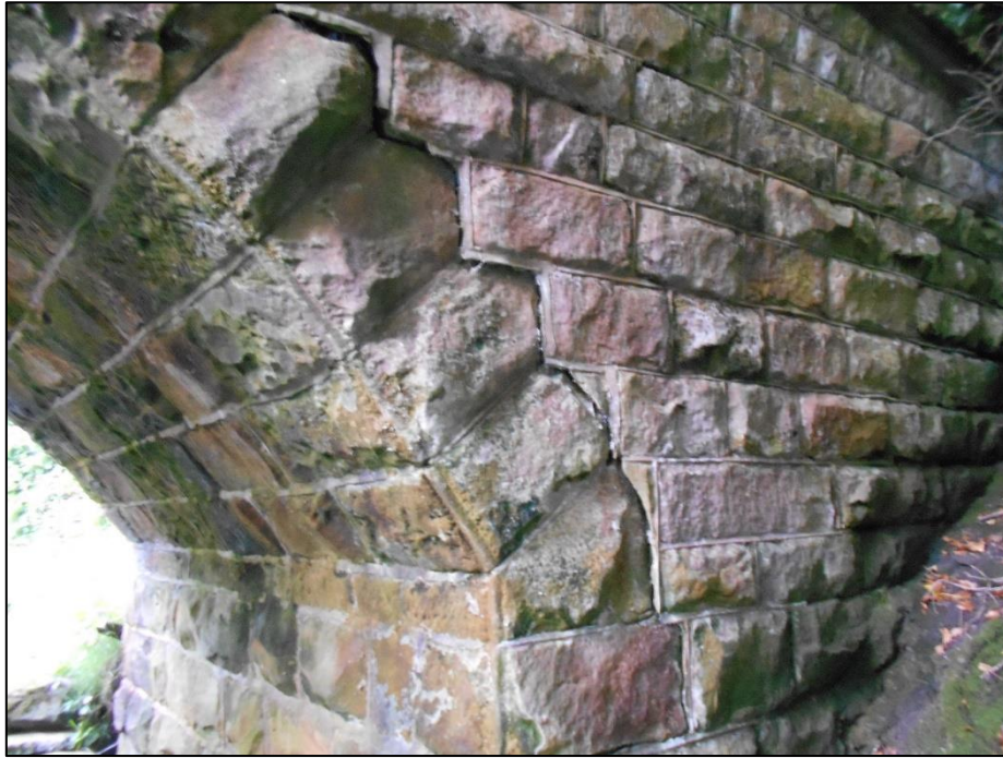
Figure 7: Substantial crack at south-west corner of bridge
