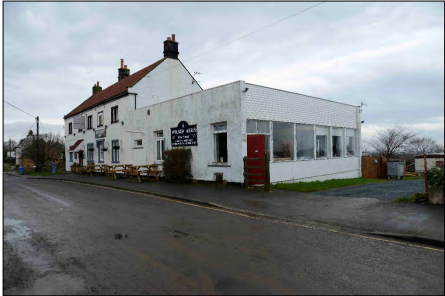
Appendix 2.4: View of the south and east elevations of the Wilson Arms, looking north-west
