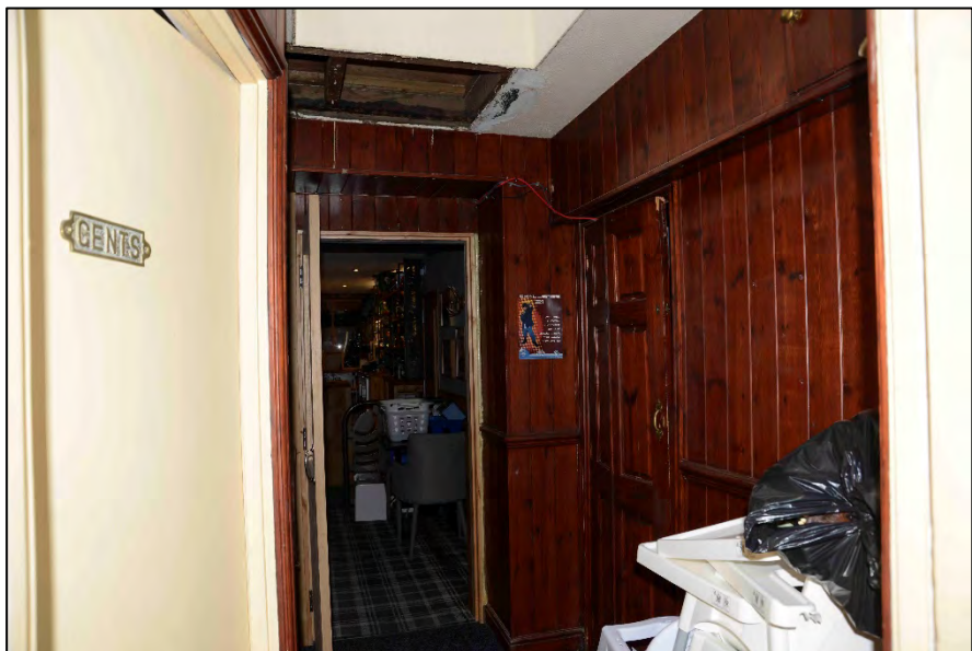
Appendix 2.9: View of the linkage between the 20 th Century extension and the historic bar room, looking west
