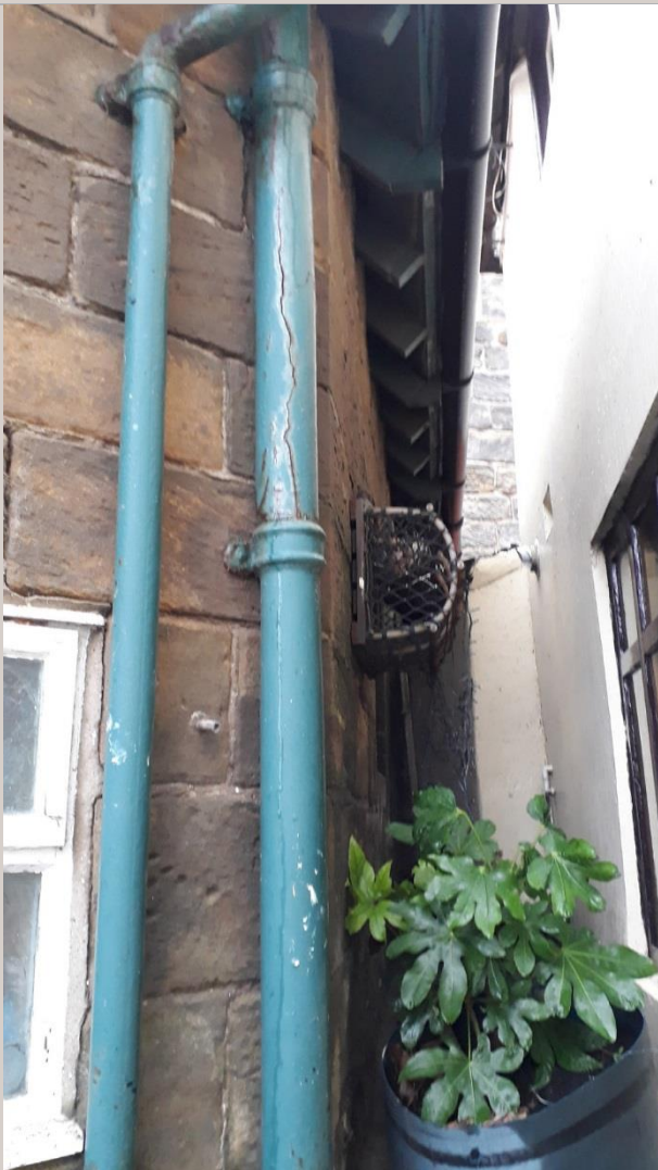
Figure 20: Detail of split in cast iron downpipe
