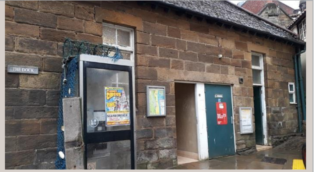
Figure 19: View to main (front) north elevation with entrances to male, female and accessible WCs and modern telephone box
