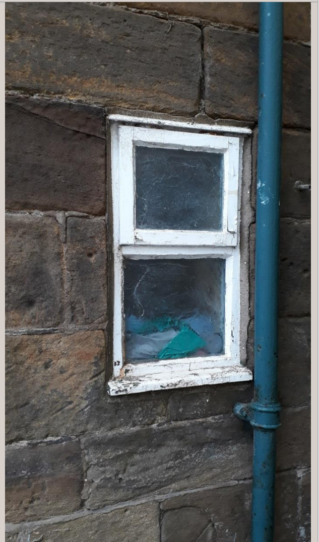
Figure 21: Example of window in need of refurbishment
