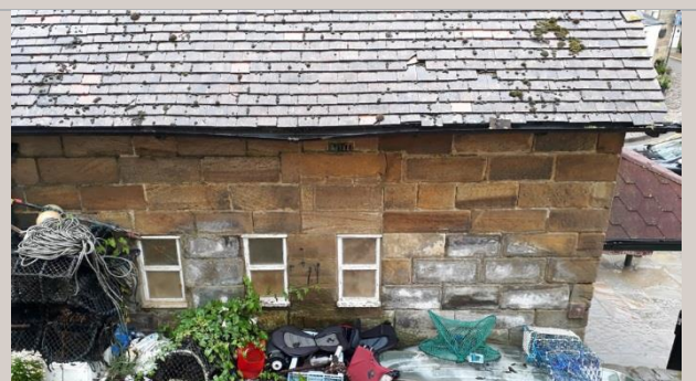
Figure 17: Detail of one of two blocked earlier windows in the south elevation. Evidence of robust stone lintel and opening infilled with stonework
