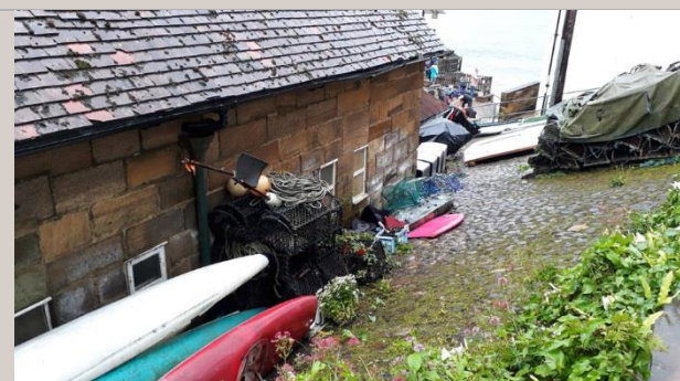
Figure 16: WC windows inserted along the south wall that faces rising ground laid with cobbled surface
