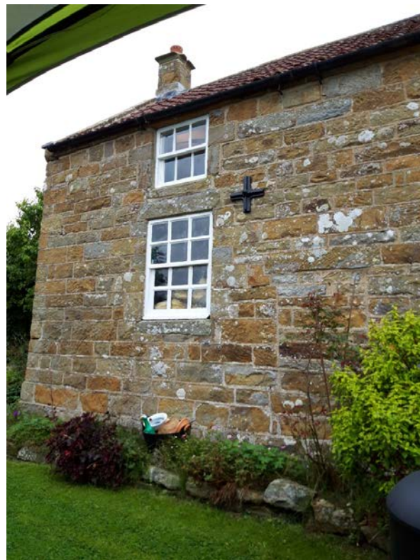
This photo shows the building on the southern gable of the dwelling, to be converted into self-contained accommodation
