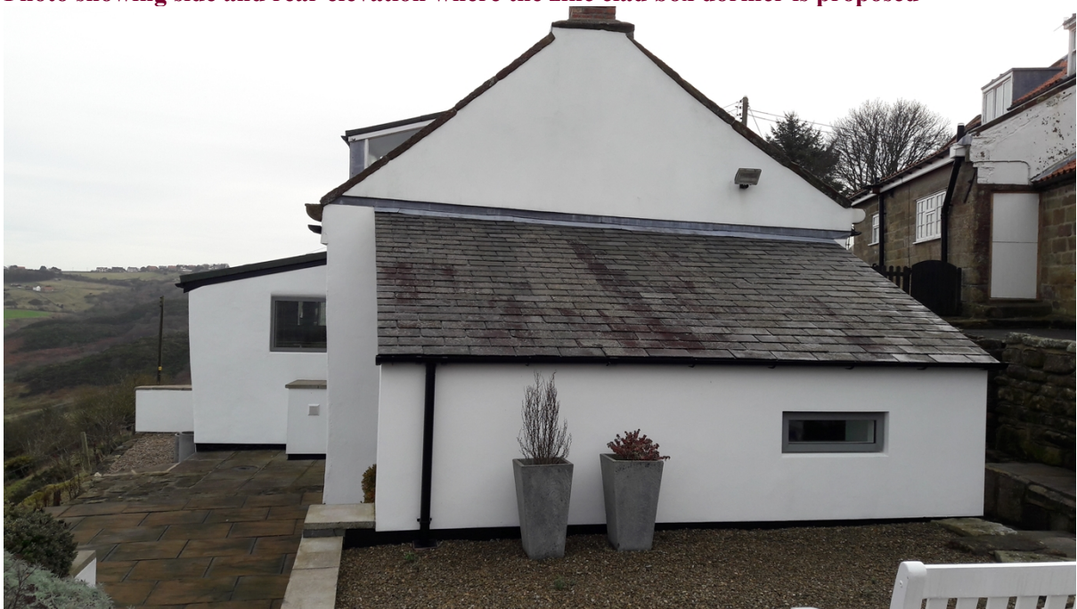
Photo showing front elevation with the existing raking dormers and lean-to extension
