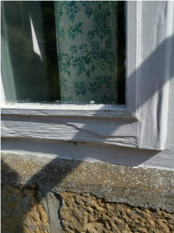
Modern casement window showing rot to casement and outer frame
