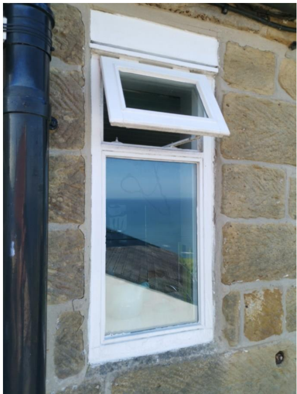
Modern casement window showing rot to casement and outer frame. Inappropriate, inconsistent design.
