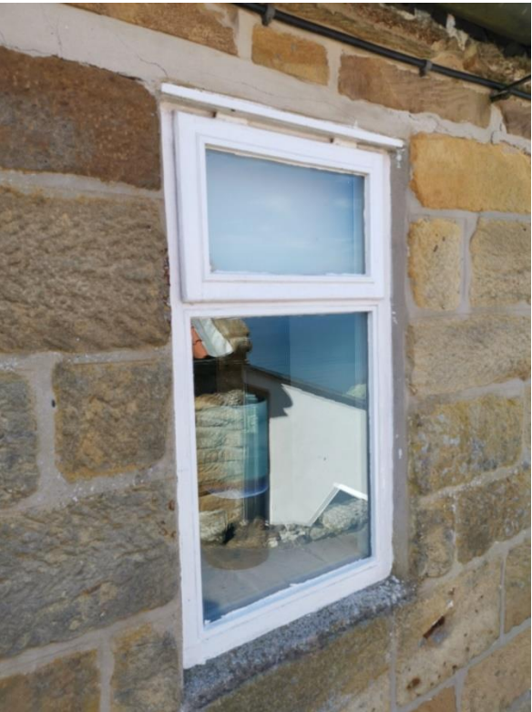
Modern casement window showing rot to casement and outer frame. Inappropriate, inconsistent design.
