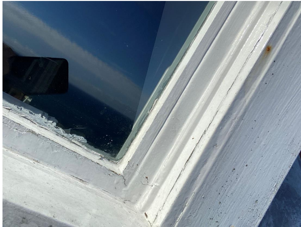
Modern casement window showing sealed double glazing to frame and decay to sill
