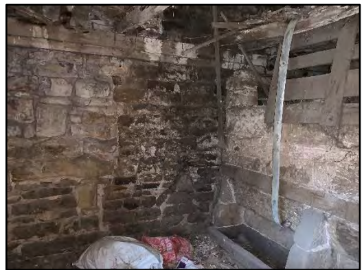
Photo 22: Inside building F; cobwebbed and damp.
