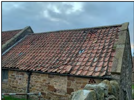
Photo 15: Missing roof tiles on building D.
