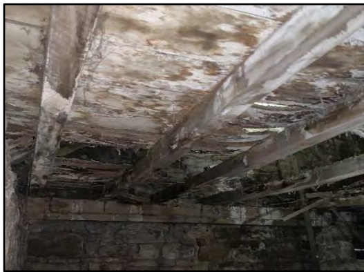
Photo 23: Cobwebbed inside of building F.
