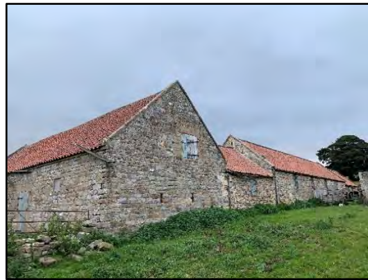
Photo 4: South-east gable end of building A and eastern aspect of building D.
