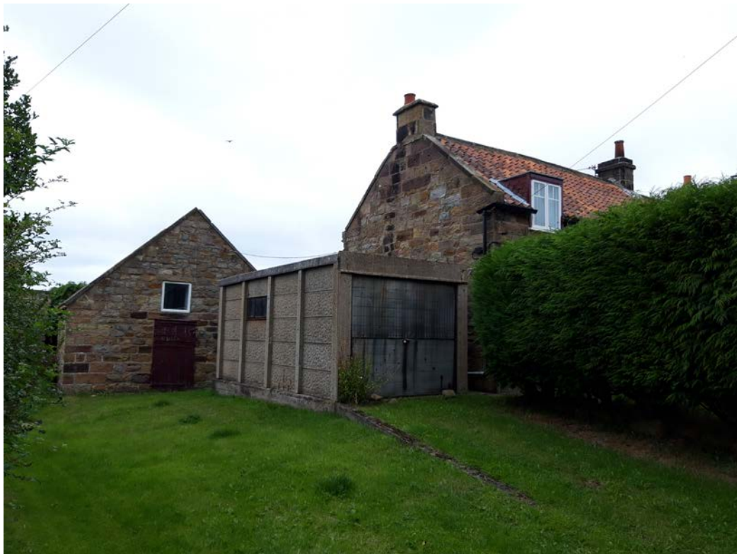
This photograph shows the gable end of the property, together with the existing garage to be replaced by the proposed two storey extension.
