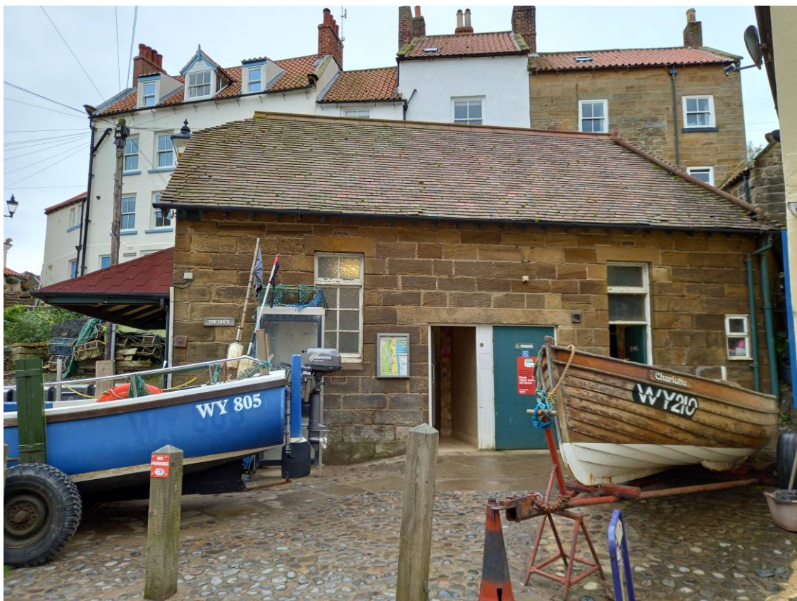
This photograph shows the north elevation roof pitch of the Public Conveniences.
