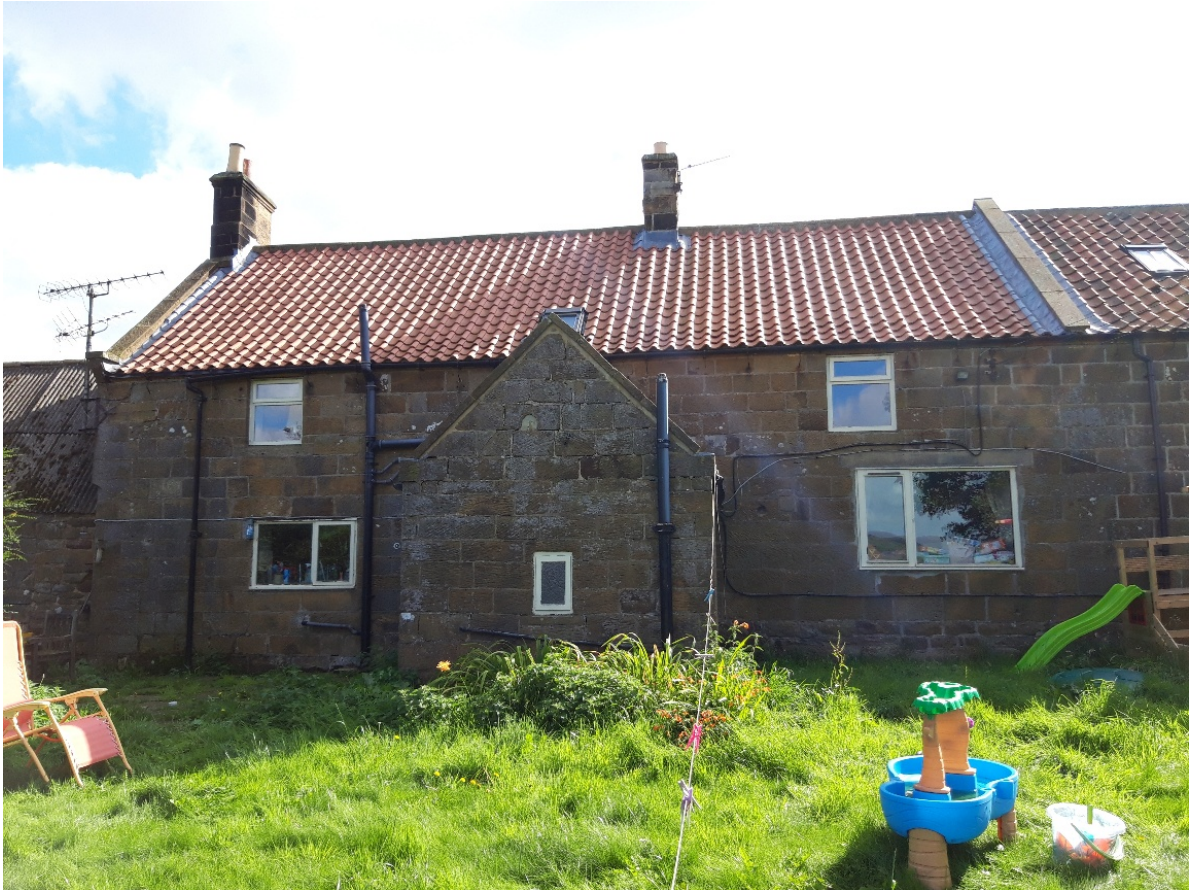
This photograph shows the rear elevation of the property, on which the proposed extension and dormer window are to be constructed.
