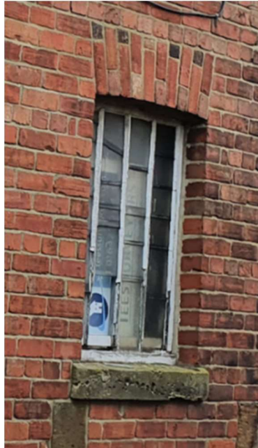
Rear window with rot in lower glazing bars
