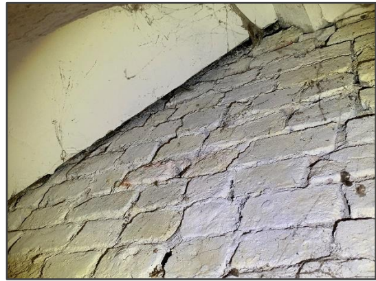
Photo 14: More internal crevices.
