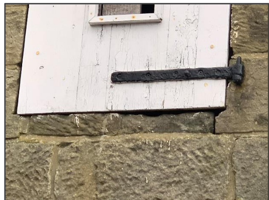
Photo 18: Large gap below outer window.
