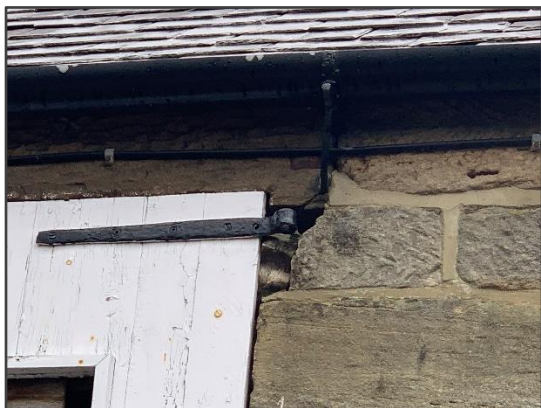
Photo 17: Large masonry crevice on southern outer wall.
