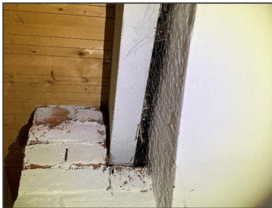
Photo 7: Gap above the internal door.
