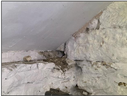
Photo 13: Large gap in stonework.
