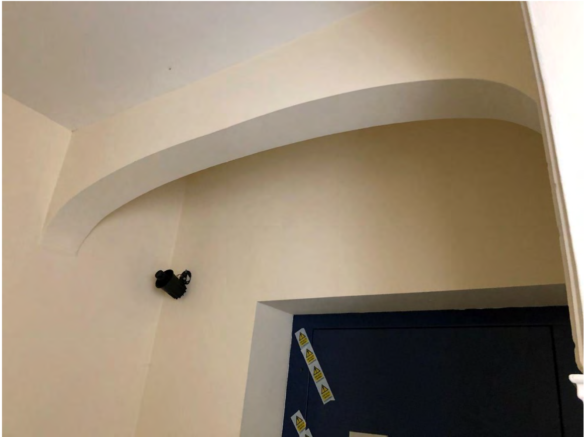
Arch in front of lift door
