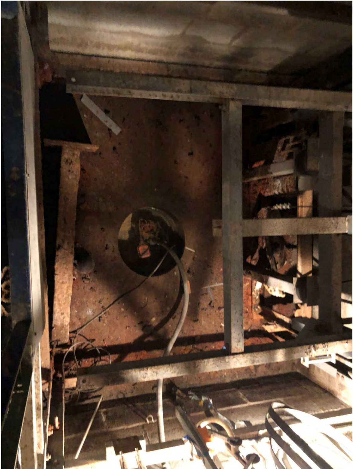
Sump and pump at bottom of lift shaft
