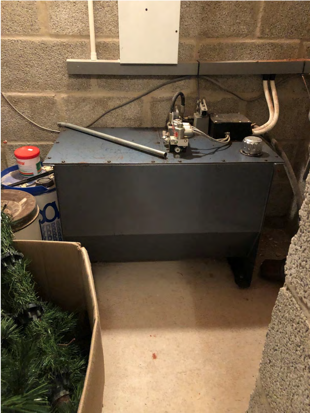
Pump for sump
