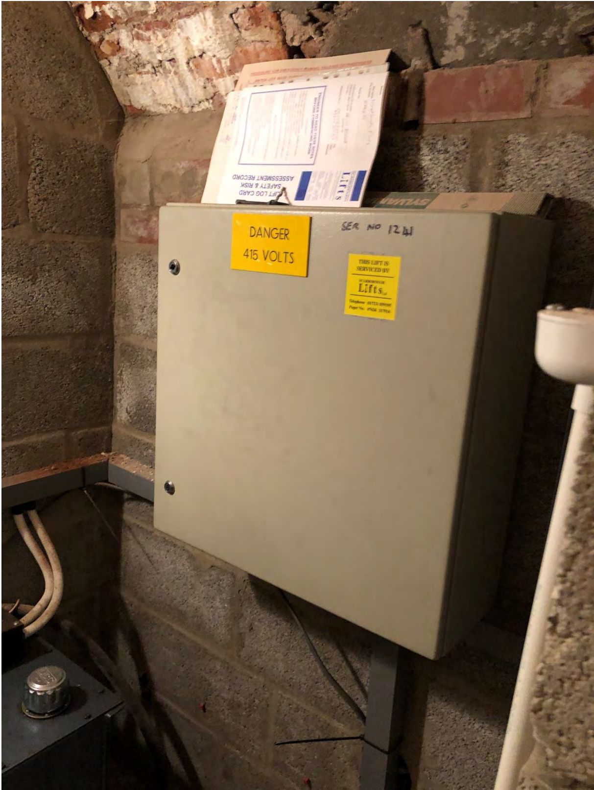
Electrical supply and switch gear
