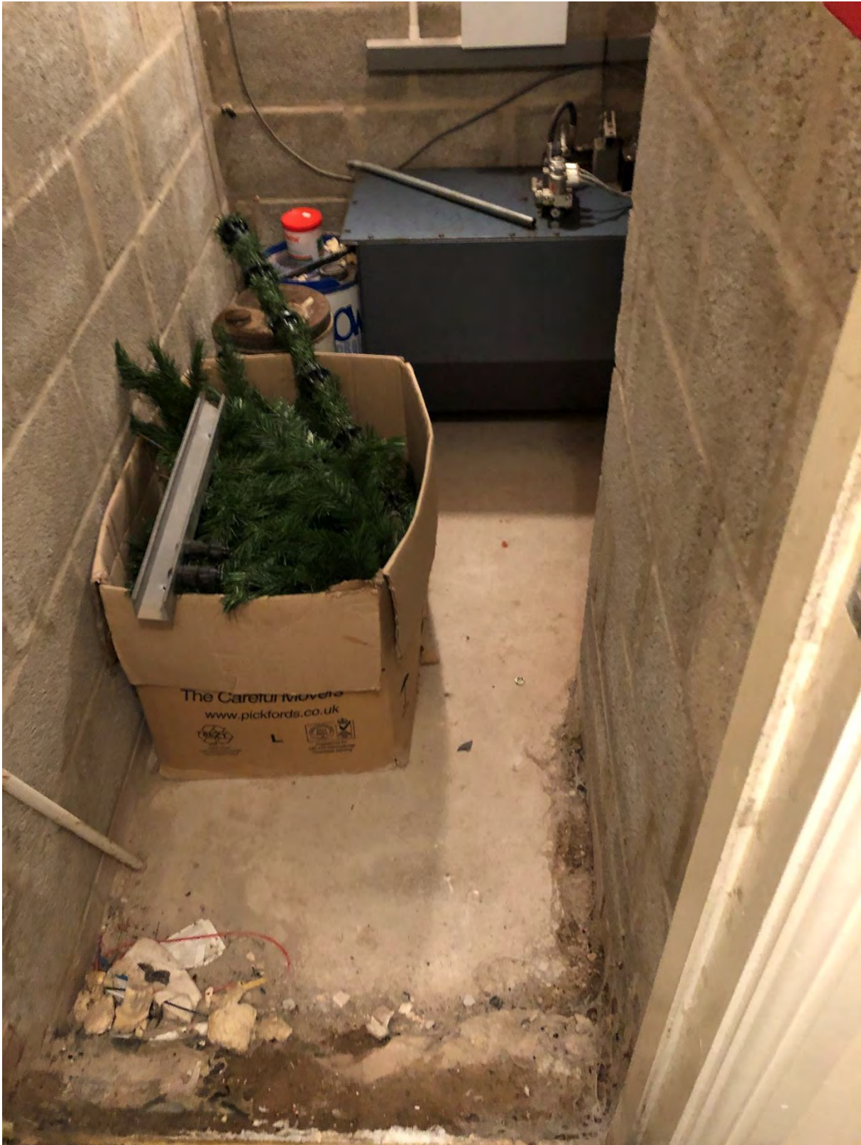
Step down into Plant room
