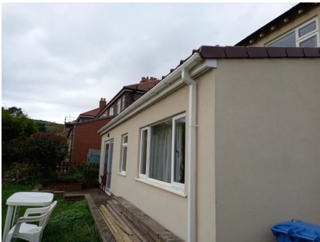
Partial view of rear elevation taken from the side drive showing the existing full width single storey lean-to extension.
