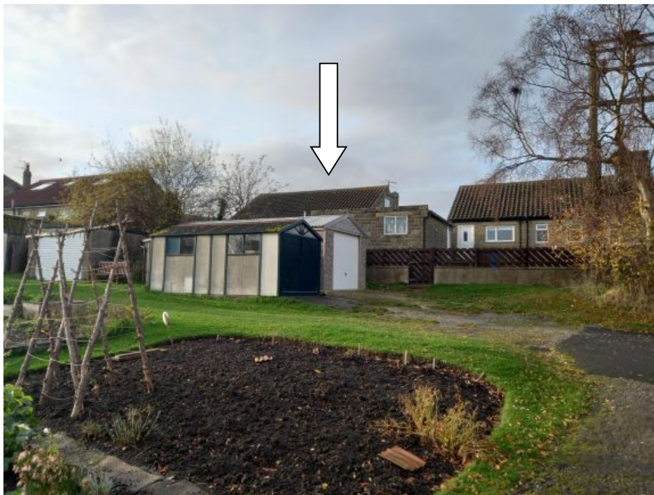
Photograph taken from allotment gardens showing the rear roofslope of the property. The roof is visible over the rooftops of two garages within the allotment gardens as identified by the white arrow.
