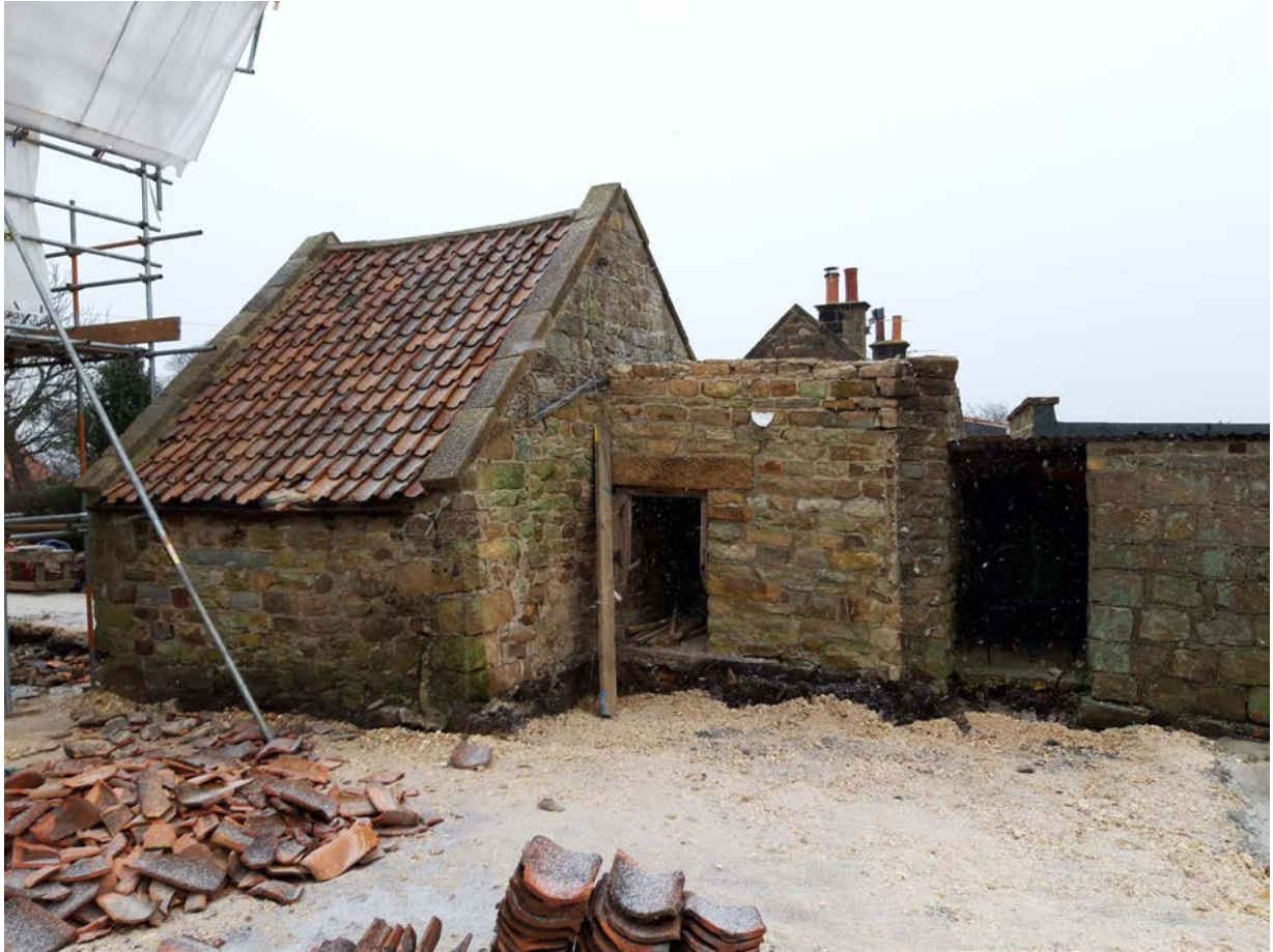
This photo shows the northern elevation of the outbuilding, viewed from within the garden.
