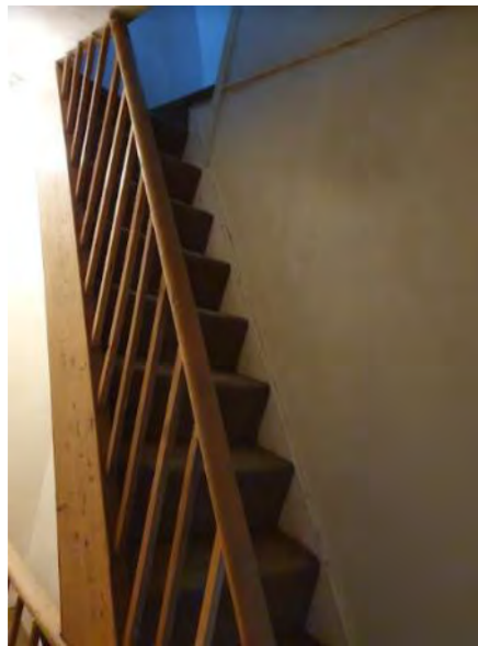
Non-historic bannister to be replaced
