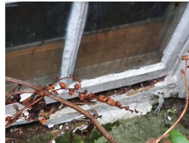
Rear windows requiring repair and repainting
