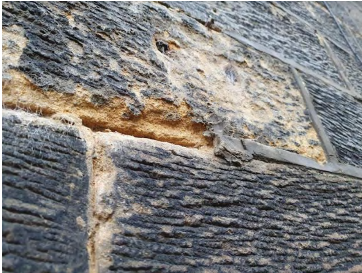
Failed cement pointing
