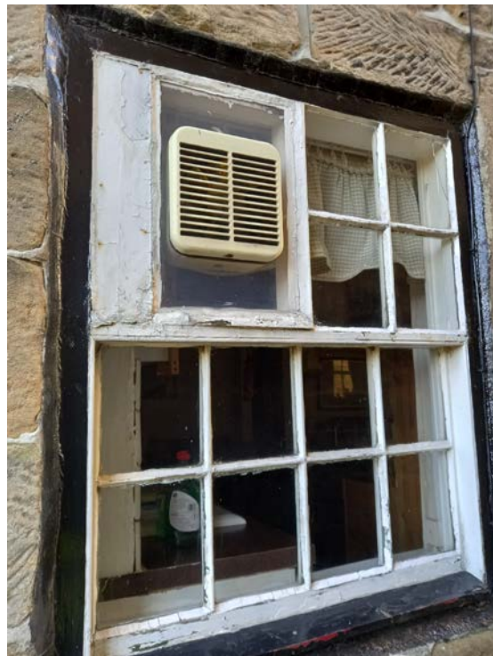
This photo shows the ground floor kitchen window to be replaced, on the south elevation.
