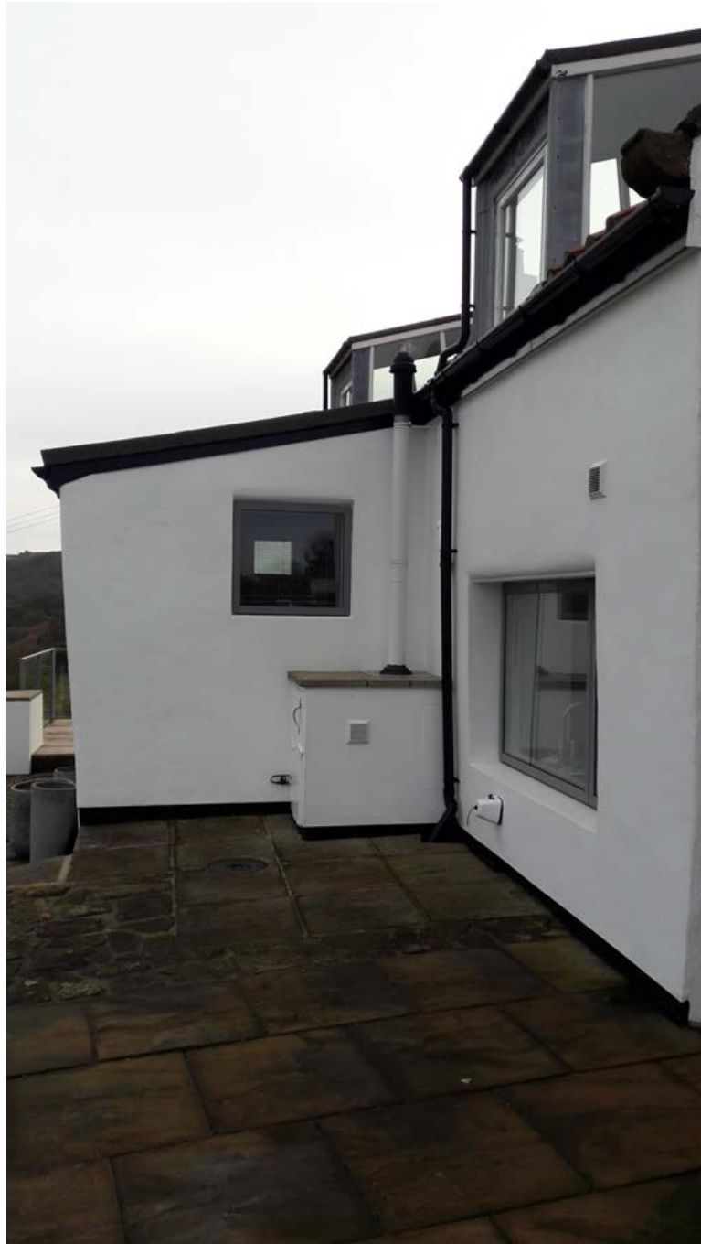
Front elevation of Susanna Hill Cottage showing the existing front lean-to projection to be built over
