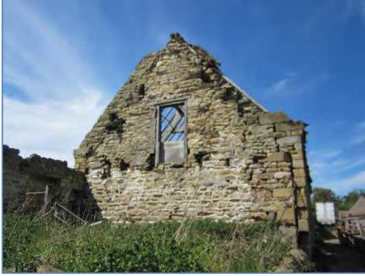
Photo 17: Building D-Crevices in gable.
