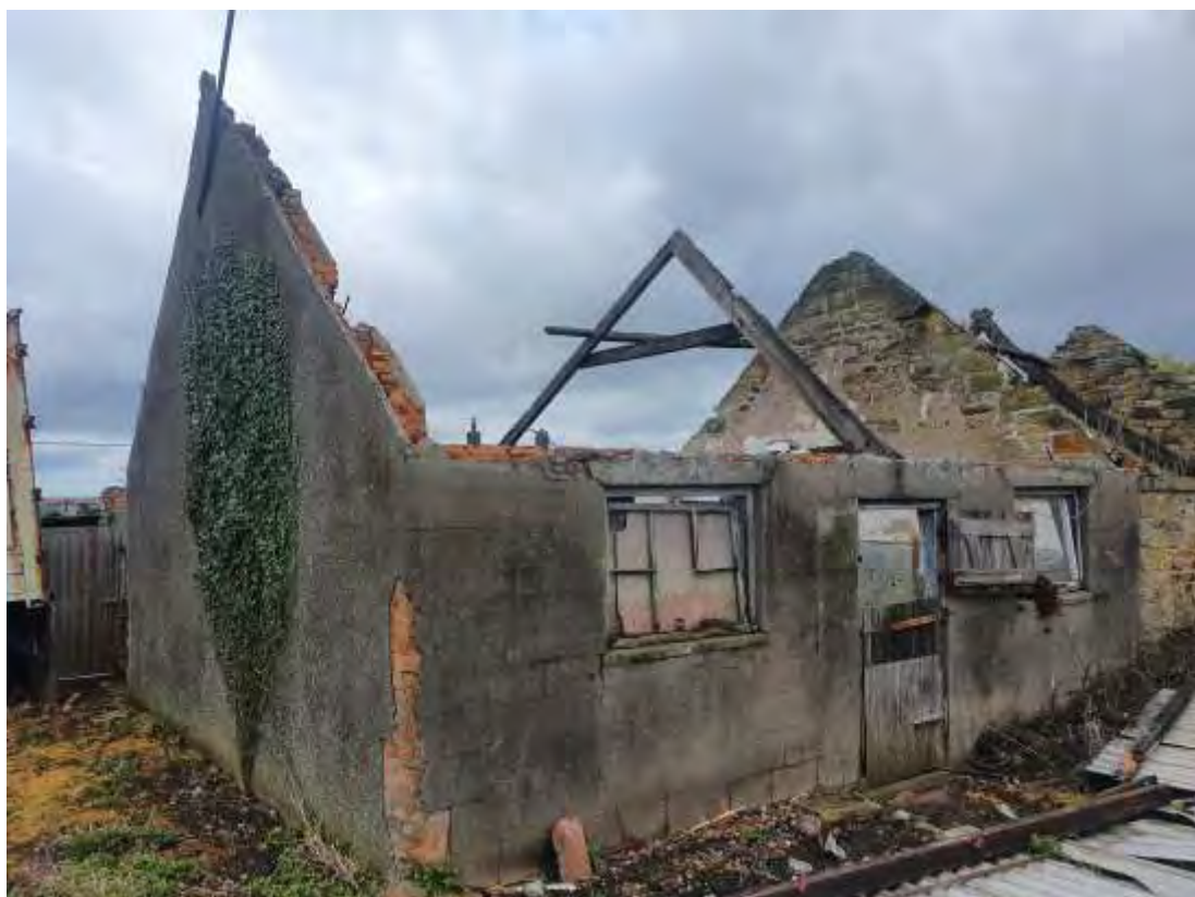
Photo 5. Rear view of the west end of the terrace. This more modern rendered brick section is to be removed.
