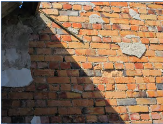
Photo 7: Building A minor crevices in brickwork..
