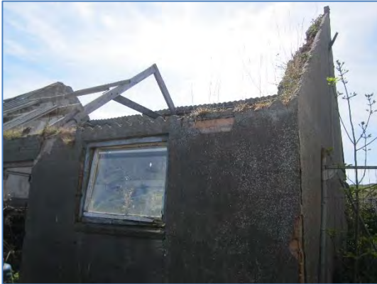
Photo 5: Building A-Missing roof.
