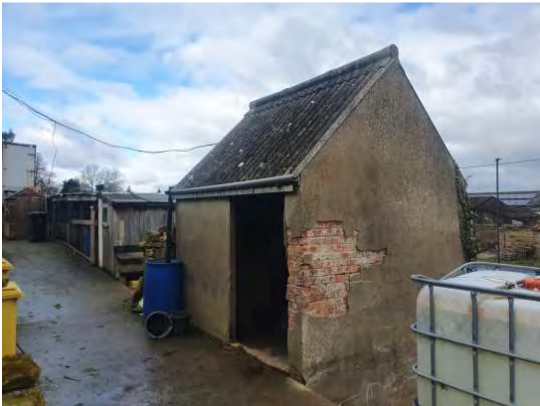
Photo 7. More modern rendered brick store to front of the main terrace to be removed.
