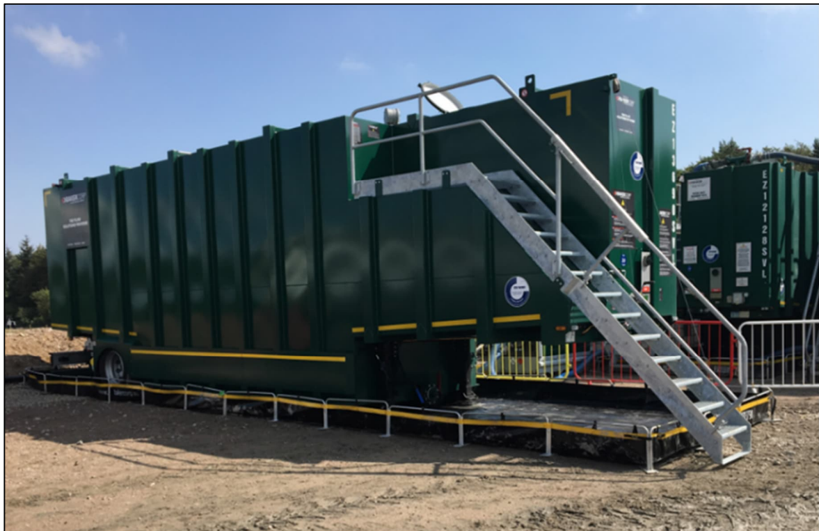
Photo 3 – Baker Tank, a similar unit will be used at Ladycross Plantation.
