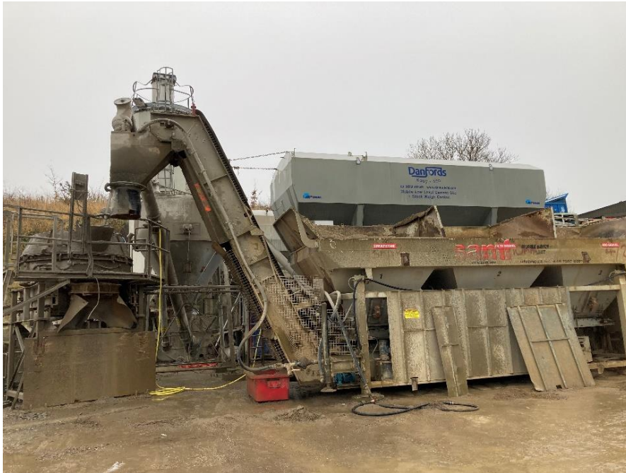
Fig 4. – Cement plant in operation.
