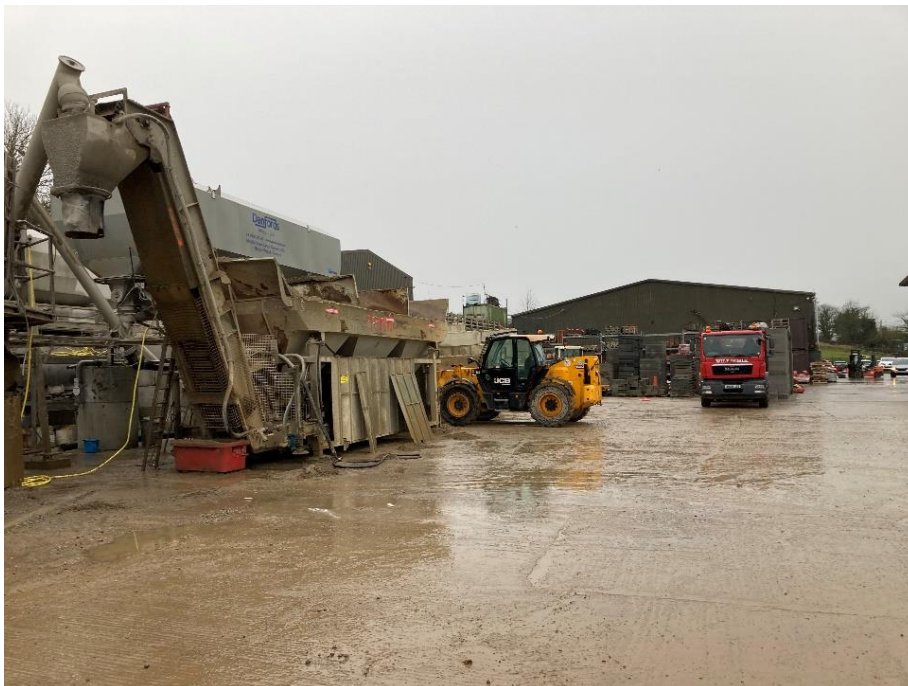
Fig 3. – Cement plant in operation.
