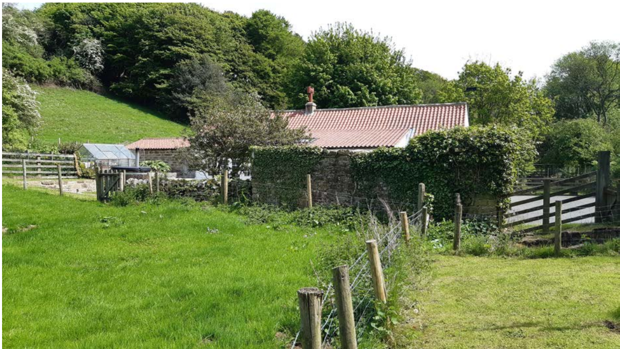
Rear elevation of North End Cottage with outbuilding for conversion to far end
