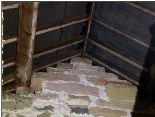
Photo 13: Lined roof in section 1c with some wall top gaps.
