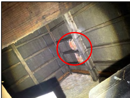
Photo 17: Large holes in lined roof of section 2b.
