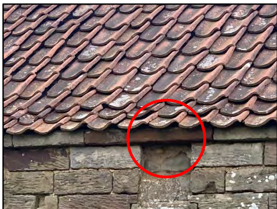
Photo 23: Large gap near eaves on west-facing aspect.
