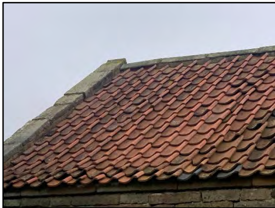
Photo 21: Some uplifted tiles on west-facing roof.
