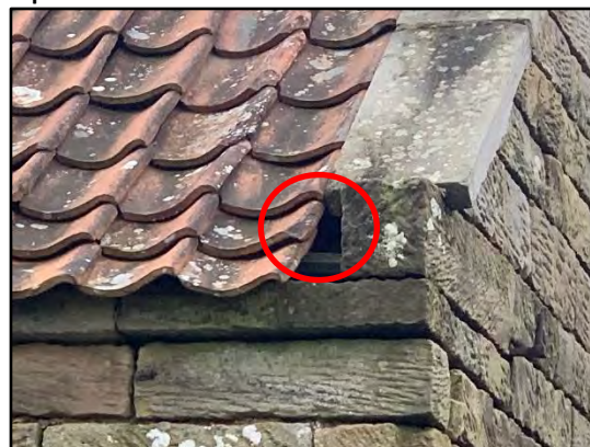
Photo 24: Large gap near corner of eaves.
