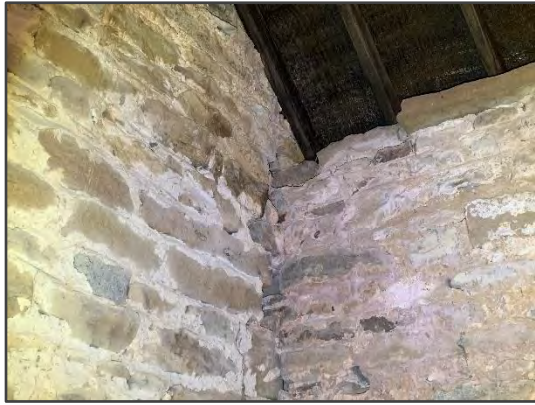
Photo 11: Masonry crevices inside section 1b.
