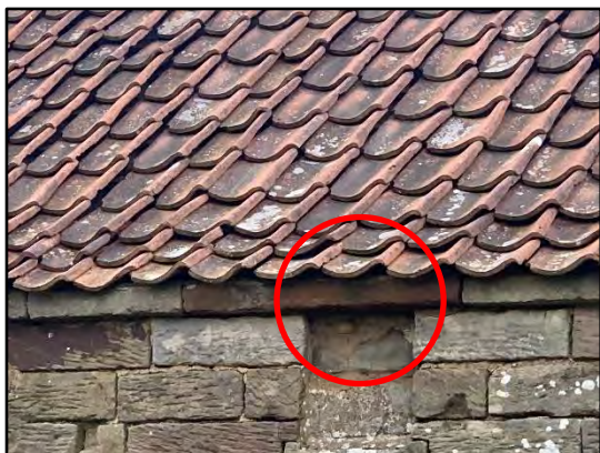
Photo 23: Large gap near eaves on west-facing aspect.
