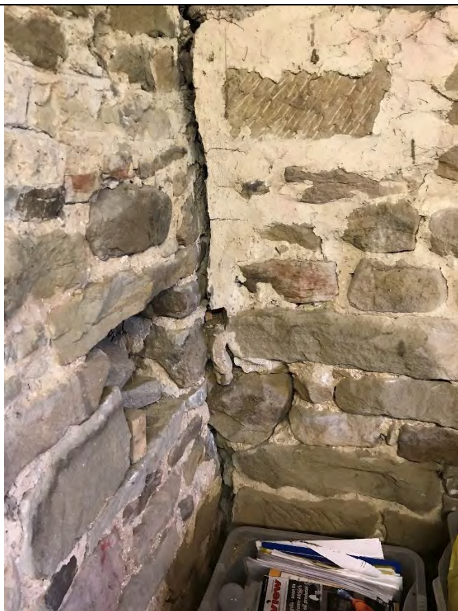
Building 1-Vertical cracking that requires remedial works
