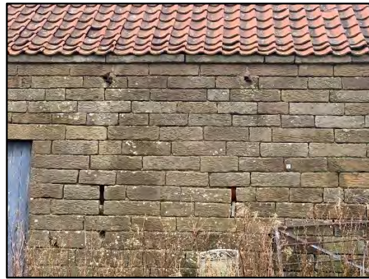
Photo 22: Some external masonry crevices on western aspect.
