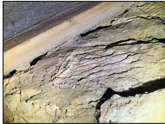
Photo 6: Wall top gaps.
