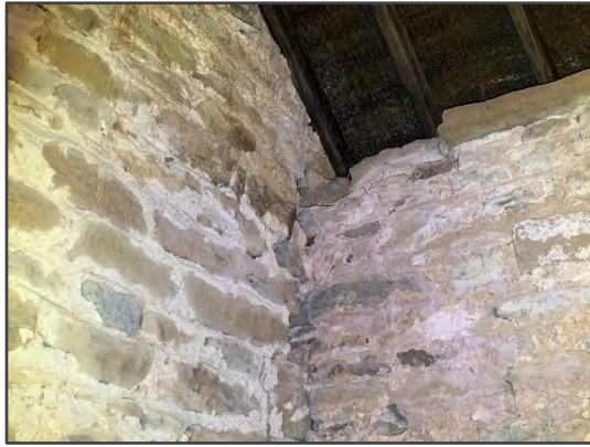
Photo 11: Masonry crevices inside section 1b.
