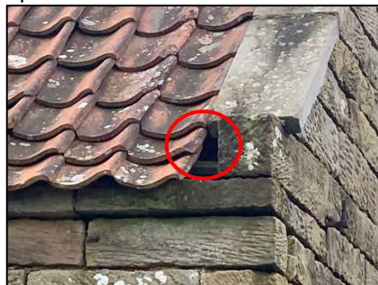
Photo 24: Large gap near corner of eaves.
