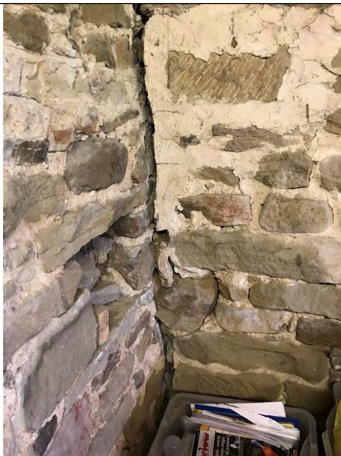
Building 1-Vertical cracking that requires remedial works
