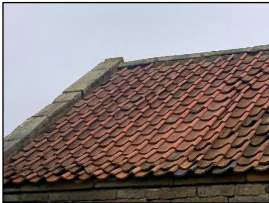
Photo 21: Some uplifted tiles on west-facing roof.
