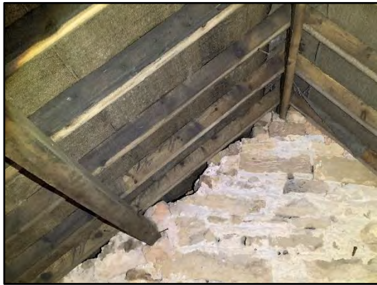
Photo 5: Bitumastic lining and large gap in section 1a.
