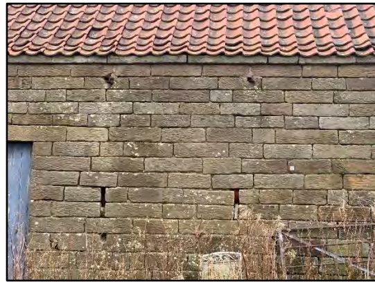
Photo 22: Some external masonry crevices on western aspect.
