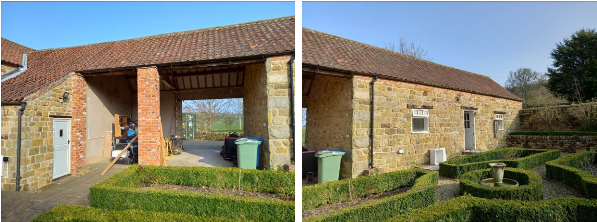
These photographs show the west elevation of Raincliffe Barn with the carport/ storage area and workspace to the right.
