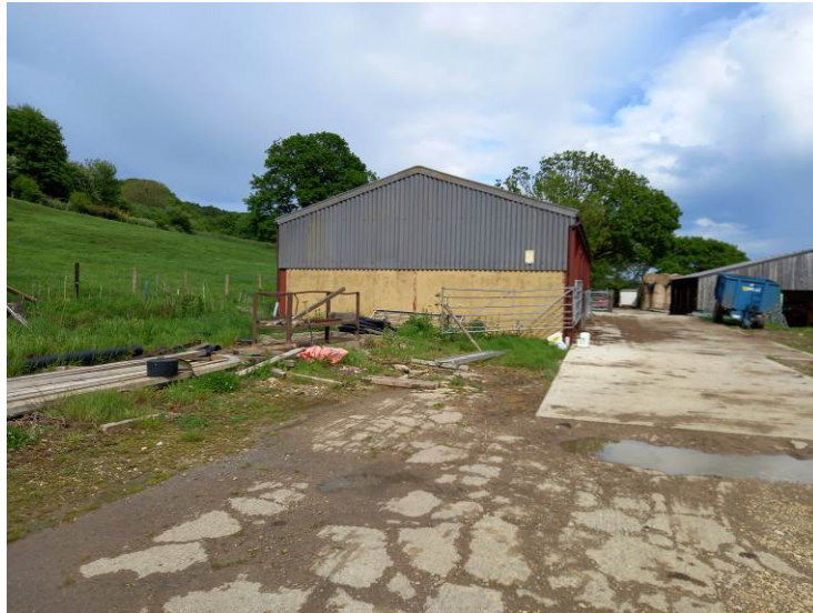
This photograph shows the proposed siting of the extension, to the west elevation of the agricultural building.
