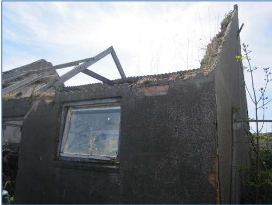
Photo 9: Building A-Missing roof.
