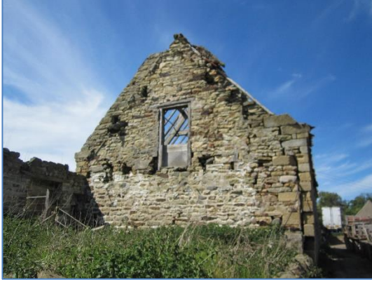
Photo 21: Building D-Crevices in gable.
