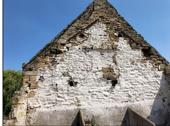
Photo 6: Gable wall crevices.
