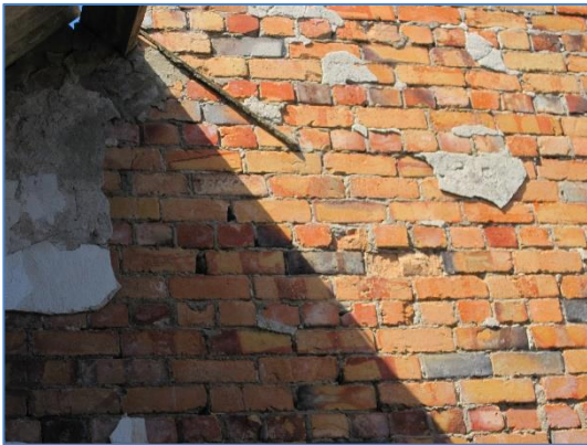
Photo 11: Building A minor crevices in brickwork..
