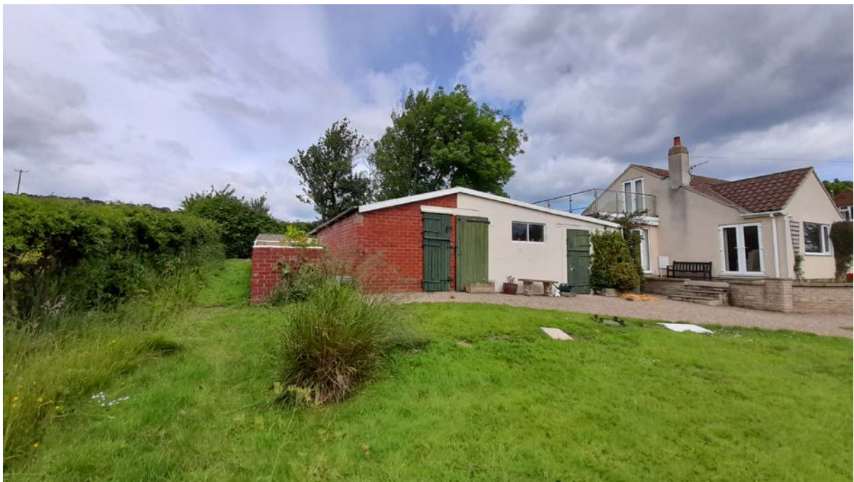
View of outbuildings and the sharp rise in land levels. The rendered section is to be removed along with the roof over
