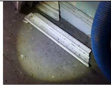
Photo 10: First floor, bat droppings
