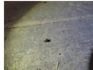
Photo 14: First floor, fresh bat droppings
