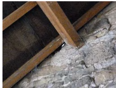
Photo 12: First floor, potential access in above bat droppings through flashing seen in Photo 5
