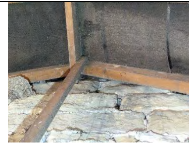
Photo 11: First floor, gaps above bat droppings
