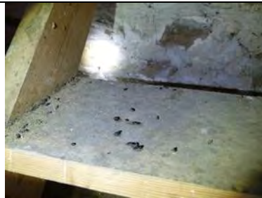
Photo 28: Fresh bat droppings on wooden ladder to first floor
