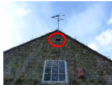
Photo 32: Hole in gable end masonry
