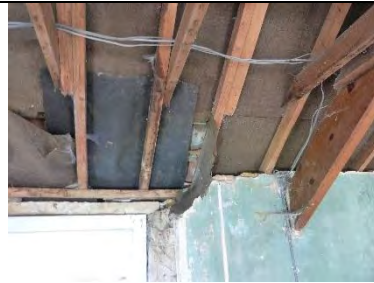
Photo 15: First floor, tares in roof lining
