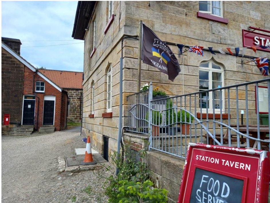
This photograph shows the front and side elevation of The Station Tavern, Grosmont. The cellar cooling unit can be seen behind the railings.
