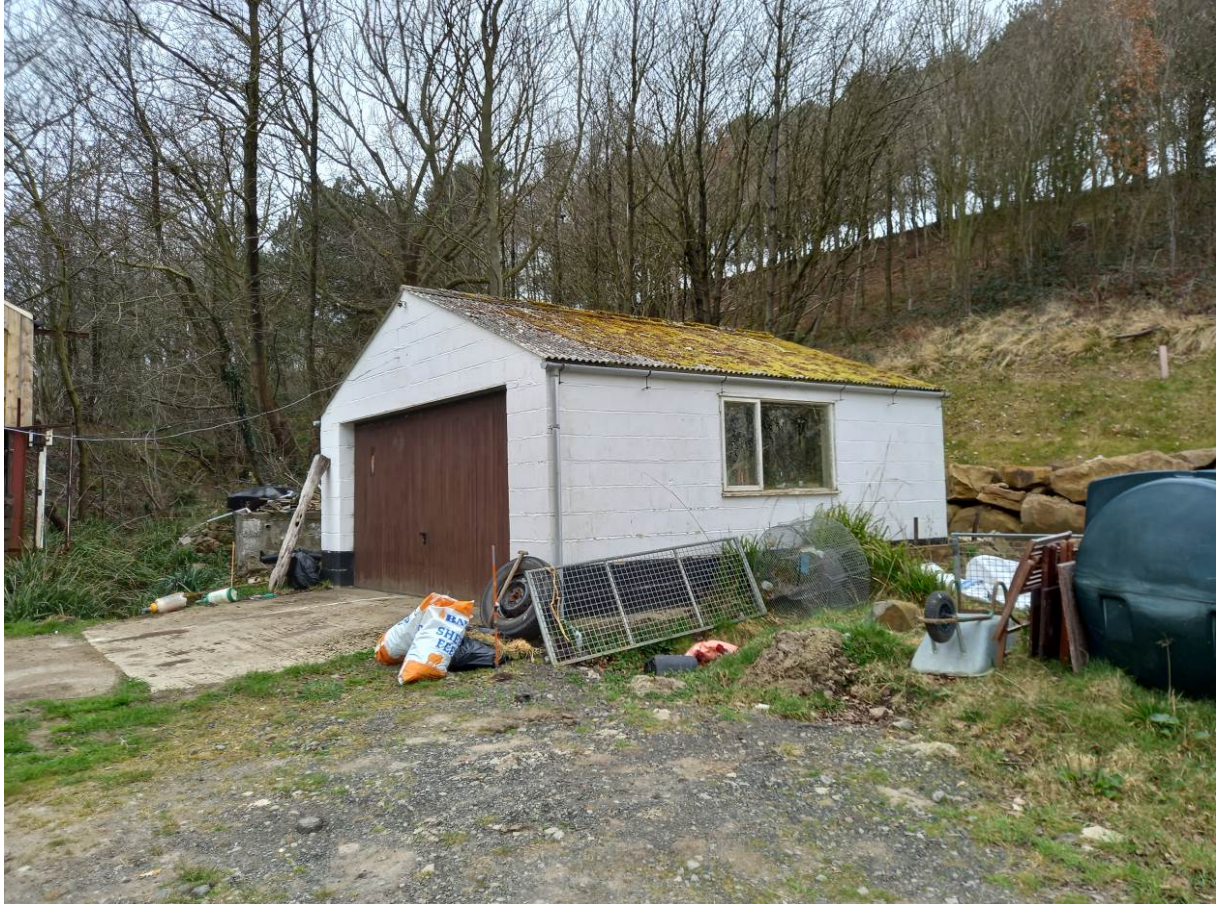
This photograph shows the existing garage to be demolished at Leith Rigg Farm, Fylingdales. The main dwelling sits opposite.
