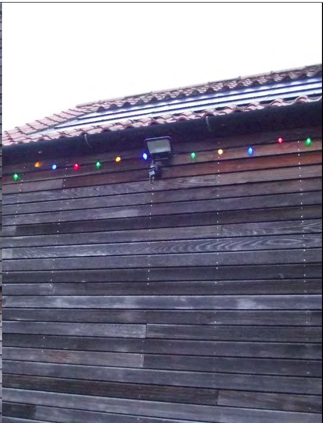
Fittings U-Location on the rear side of building within the courtyard
