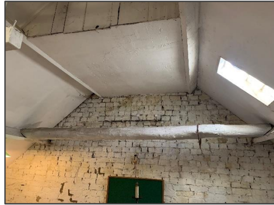
Photo 12: Masonry crevices on eastern gable wall.
