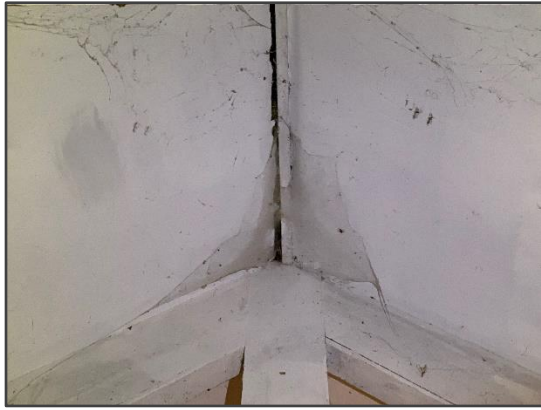
Photo 11: Gaps along internal ridge beam.
