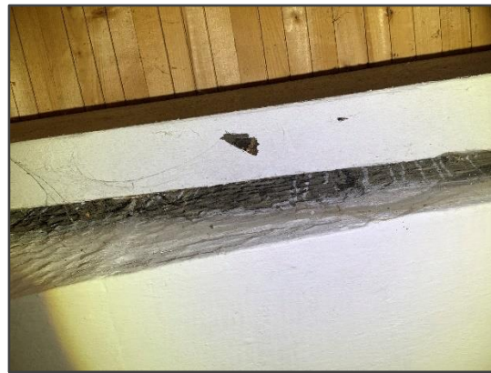
Photo 8: Wall top gap.
