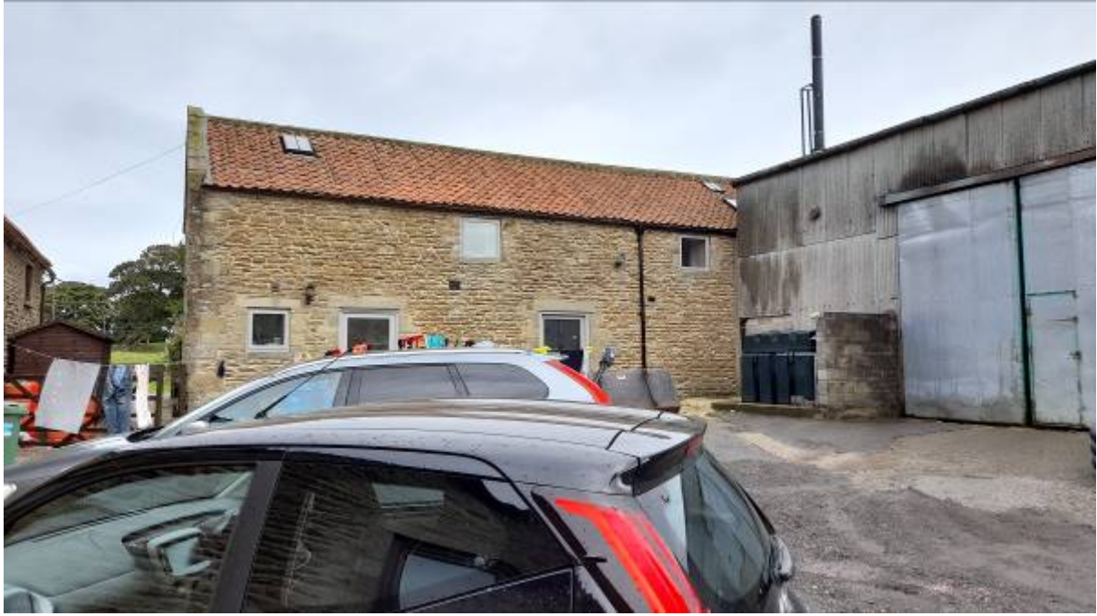
Front Elevation of Existing Barn with Modern Barn Attached and Covering a Proportion of the Building
