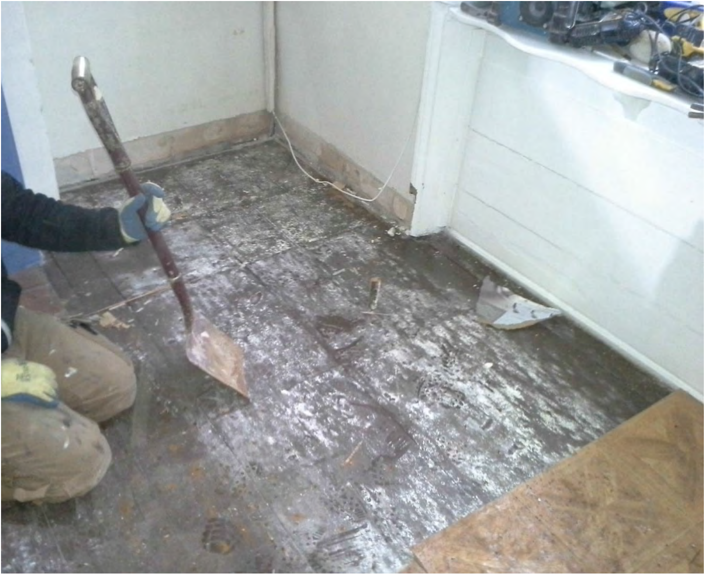
Photo shows the scale of rot to sections caused by moisture in the cellar and Dry / Wet Rot. Unfortunately, photos are lacking this week which would have helped in proving everything raised beyond doubt.
