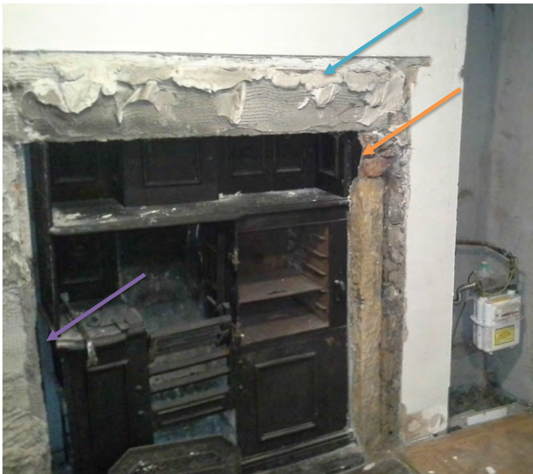
Photo 3. The Poorly fitting non original Range and evidence of previous alterations
