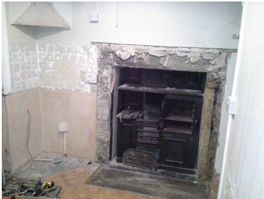
Photo 2. The non-original poorly fitting range after removal of non-original stone surrounds installed by others in 1970'
