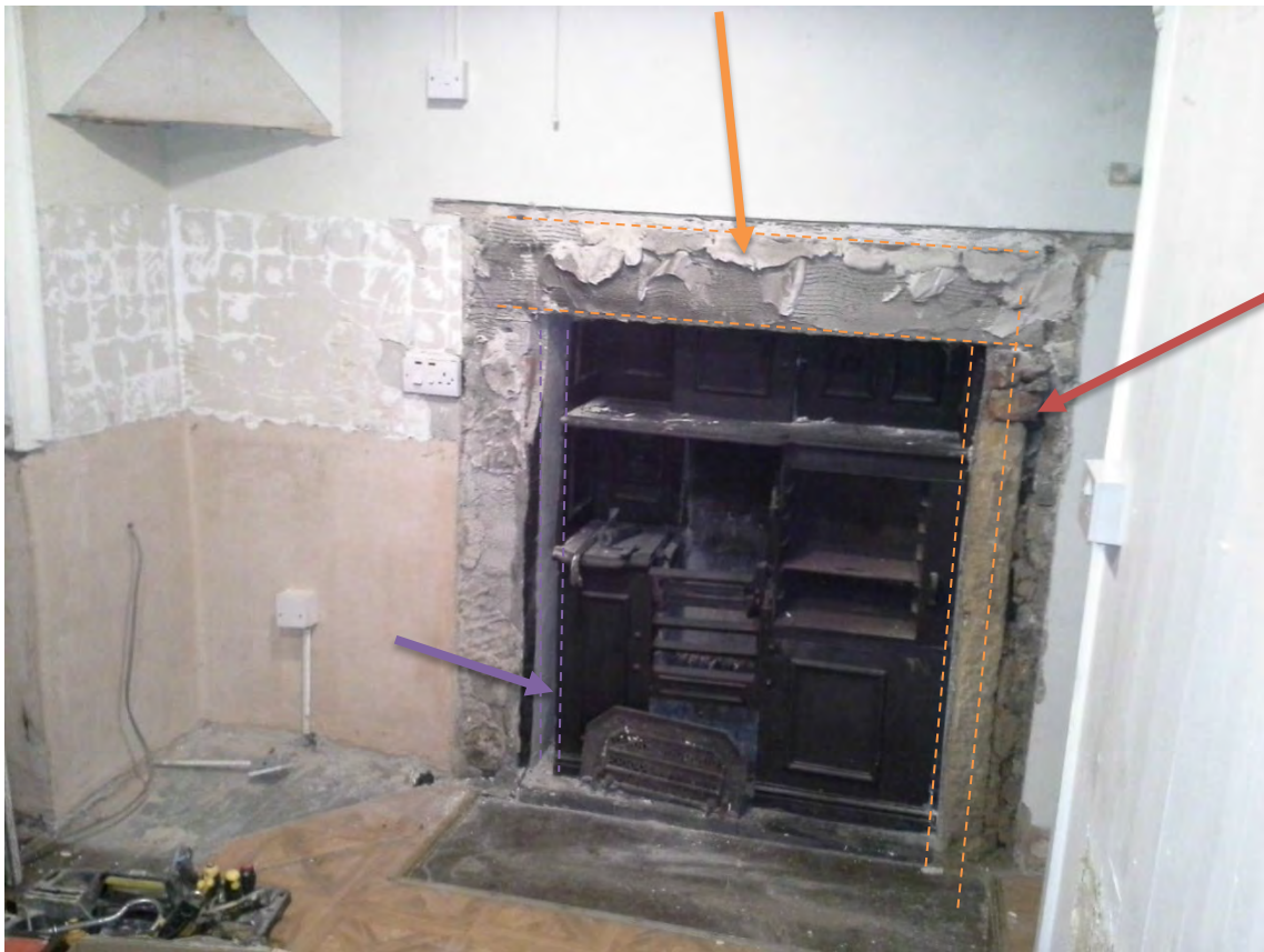
Photo 4. The Poorly fitting non original Range and evidence of previous alterations
