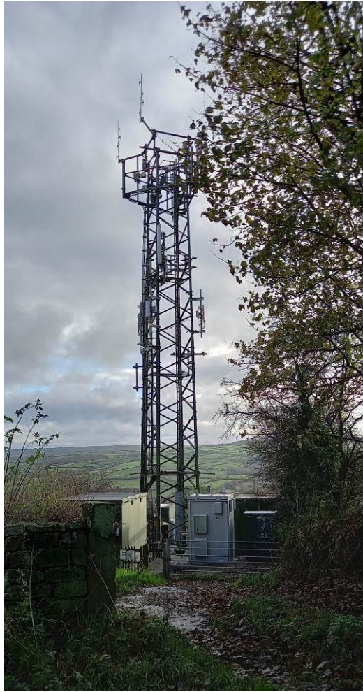
This photograph shows the mast as existing, photograph taken looking towards the south east.
