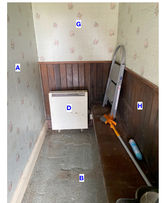
fig 11: retain existing timber panelling and bench. Strip out carpet, storage heater, stud walls, wallpaper and ceiling.
