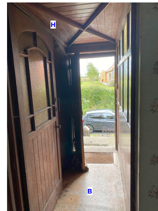
fig 10: existing timber panelling to north wall, lobby ceiling and lobby door to be retained.
