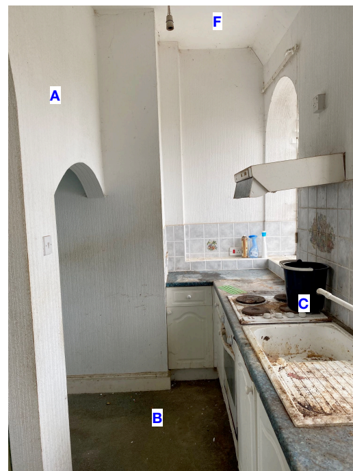
fig 8: strip out existing kitchen fittings, ceilings, stud walls, floor finishes and services.
