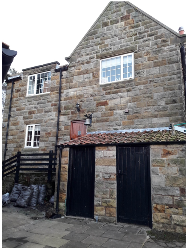
This photo shows the elevation on which the proposed porch is to be constructed.
