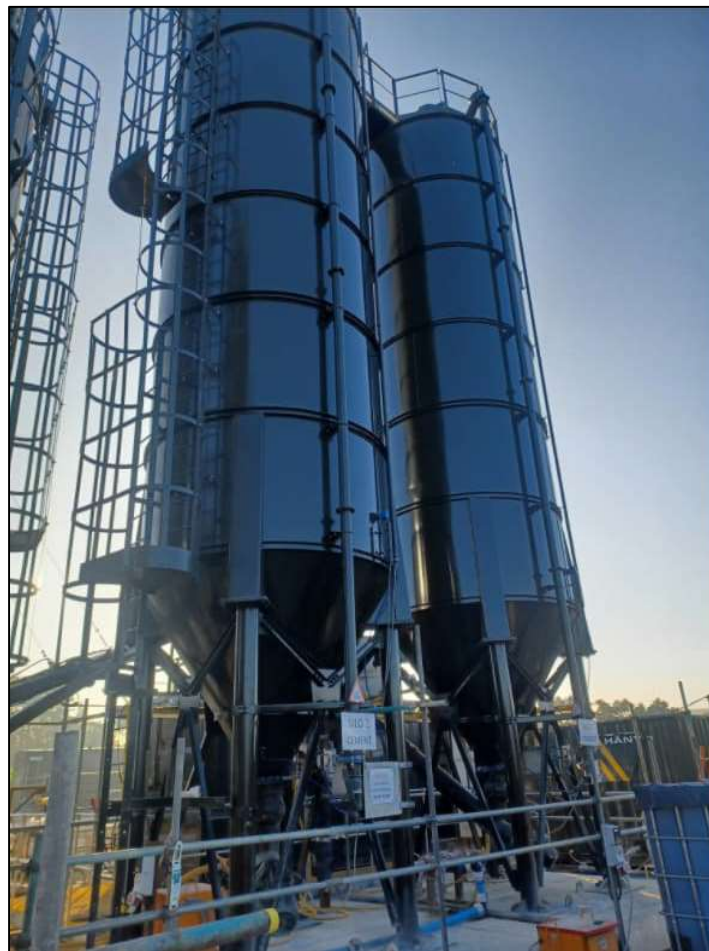
Image 14 – Grout batching plant silos
