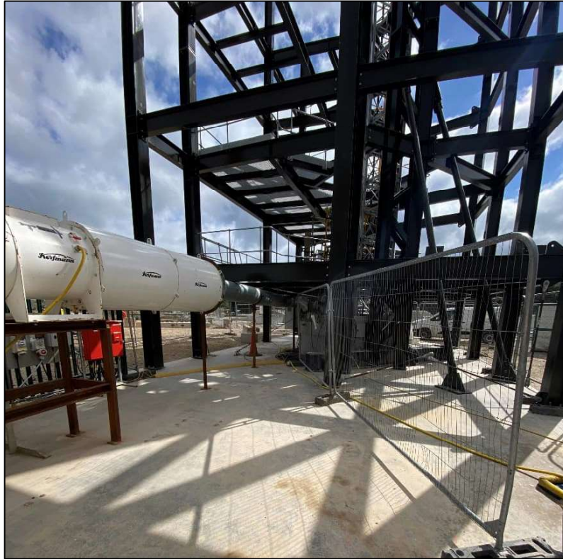
Image 3 – Shaft ventilation fan as installed at the Lockwood Beck Site.
