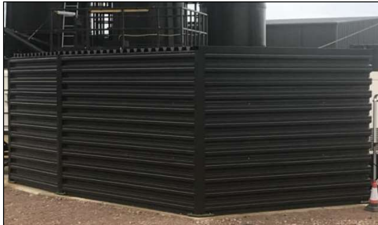
Image 2 – Emergency winch and generator shelter
