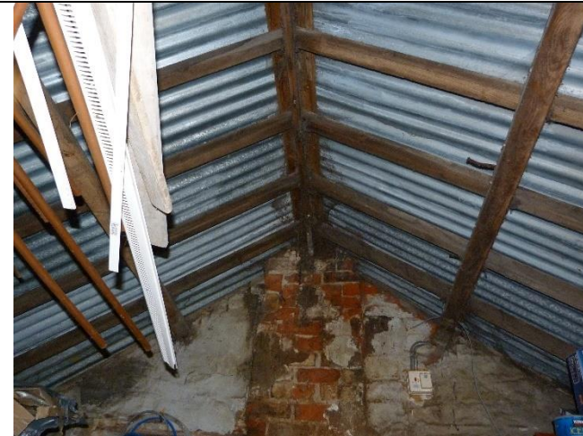
Photo 5: Internal view of the roof of the gabled section. Cobwebs evident at ridge.
