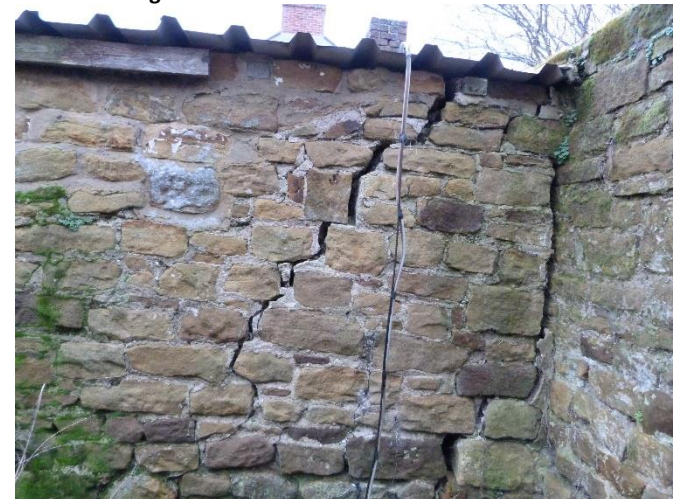
Photo 8: North wall of the building with large masonry crevices.
