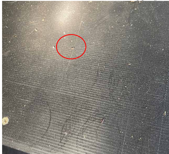
Plate 14 – Unit 3, internal, bat droppings.
