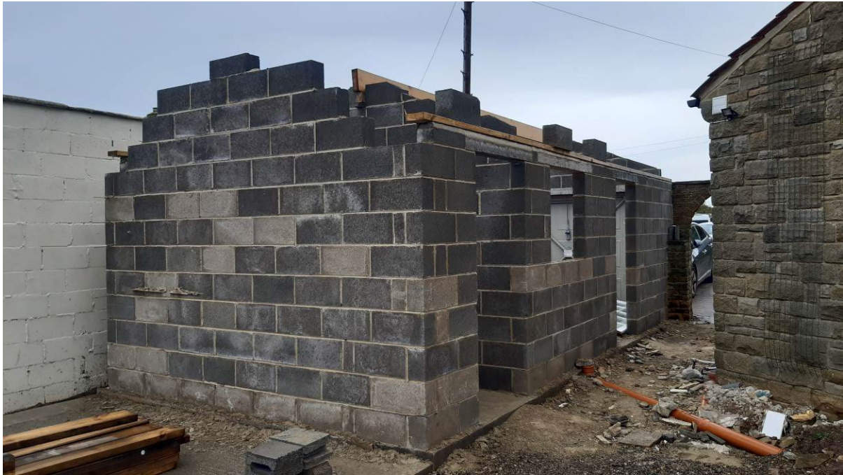
Rear view of the store/dog grooming salon under construction in place of the former concrete sectional garage
