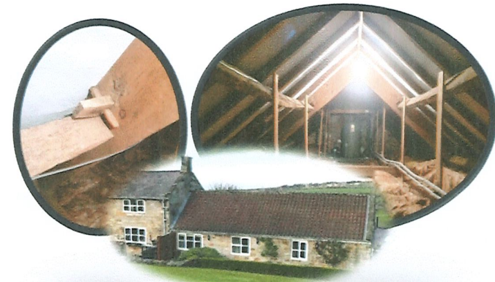
Historic purlin traditionally joined into modern truss, present in the earliest barn
