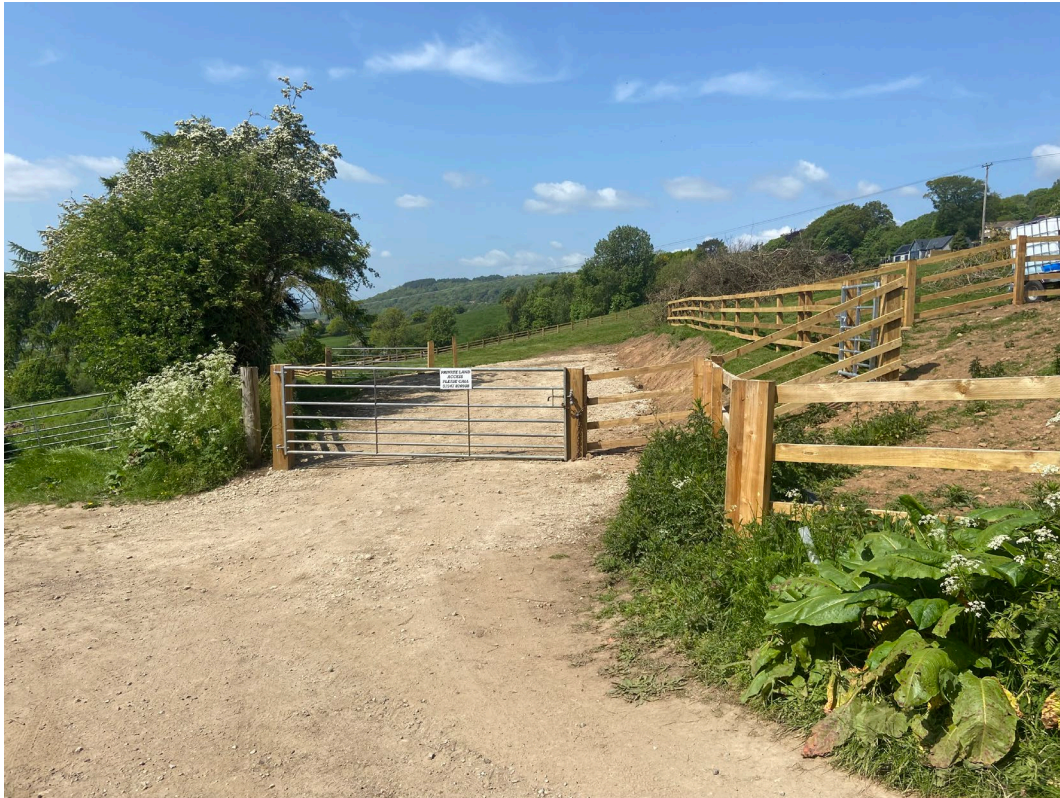
This photo shows the new access that has been created to serve the proposed stable, together with the unauthorised groundworks.
