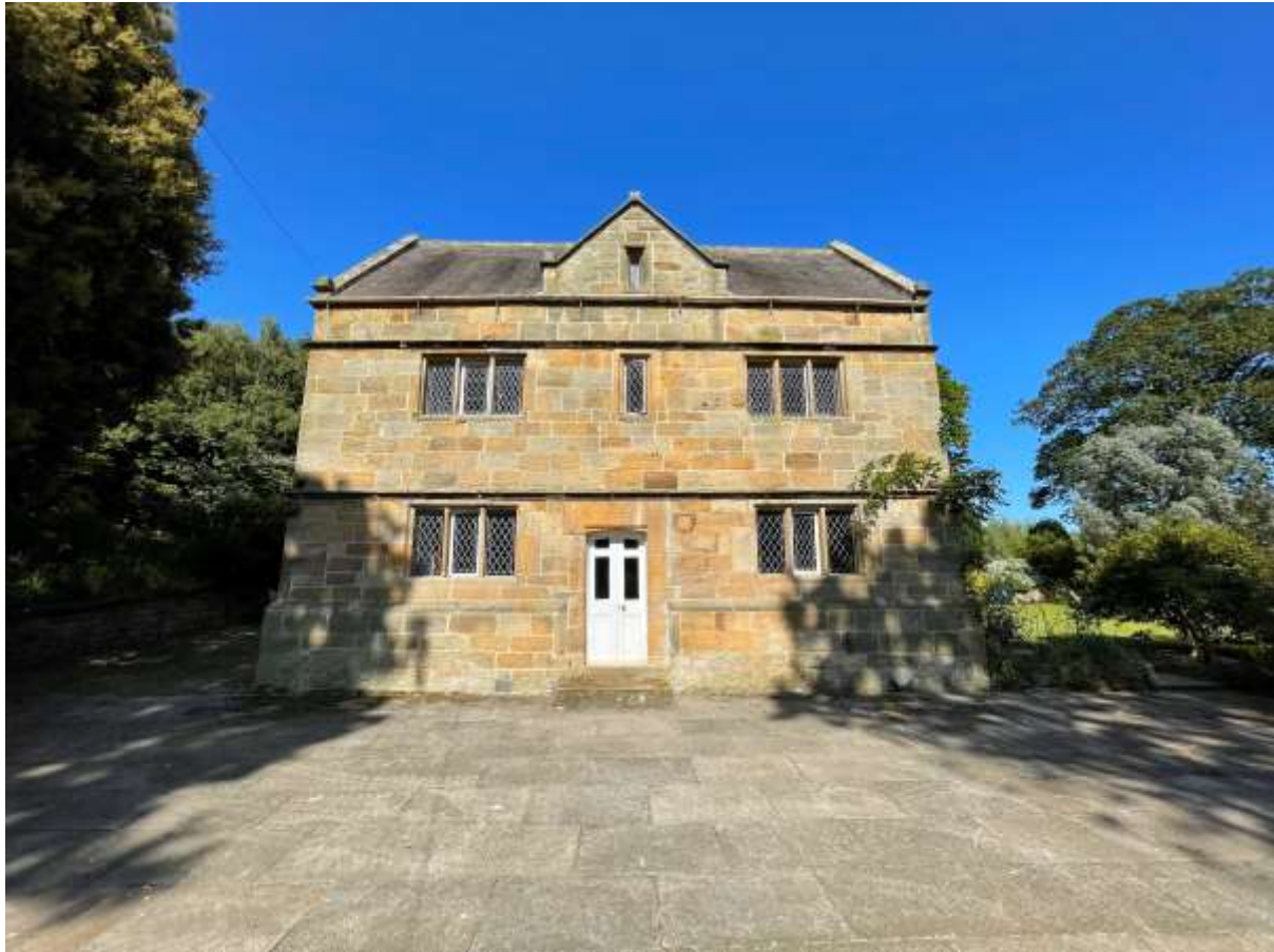
Figure 18 - Southwest facing elevation of 'Original House'. Terrace to be renewed. Existing guttering to be removed and replaced with new profile guttering running towards new downpipe.
