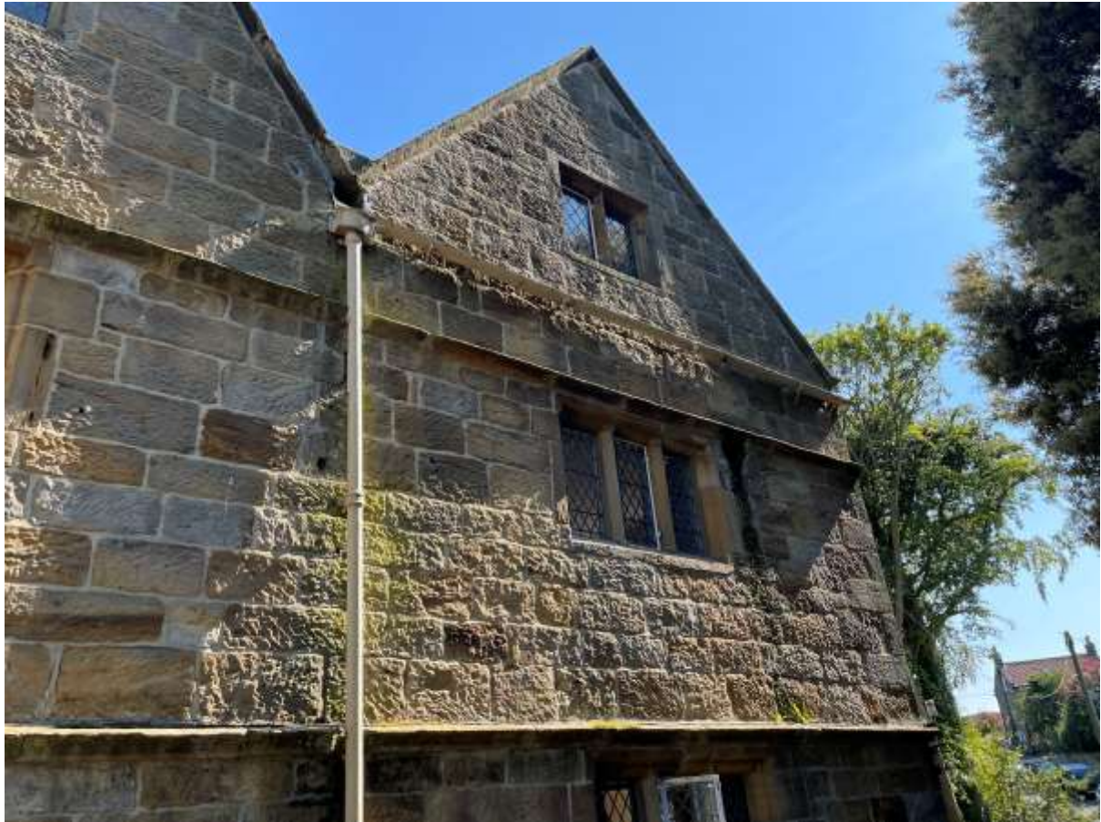
Figure 16 -Northwest Elevation of 'Original House'. Horizontal guttering above first floor level to be removed with new downpipe installed to northwest / southwest corner. Existing valley downpipe to be renewed.
