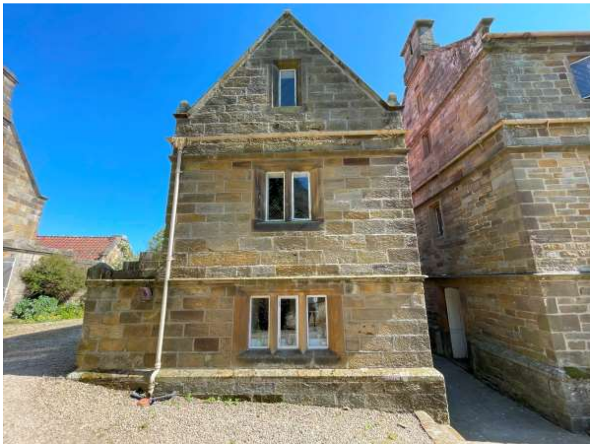
Figure 13 - Northwest Facing Gable (c.1844). Horizontal Gutter at first floor level to be removed. Downpipe to be renewed.
