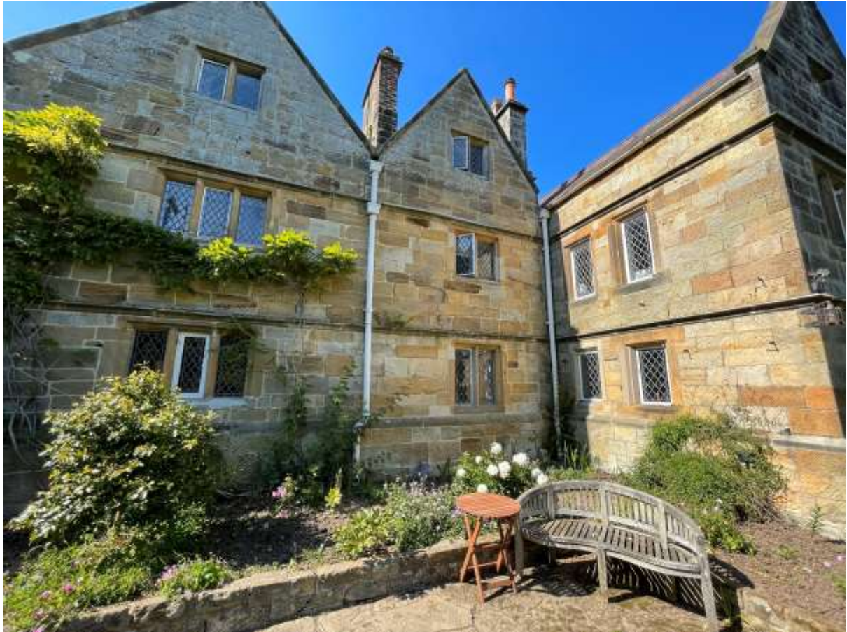
Figure 19 - Southeast facing elevation of 'Original House' and Southwest side elevation of 1835 extension. Valley downpipes to be removed and replaced with new, including hoppers. Guttering to 1835 extension to be renewed with new profile cast iron guttering.
