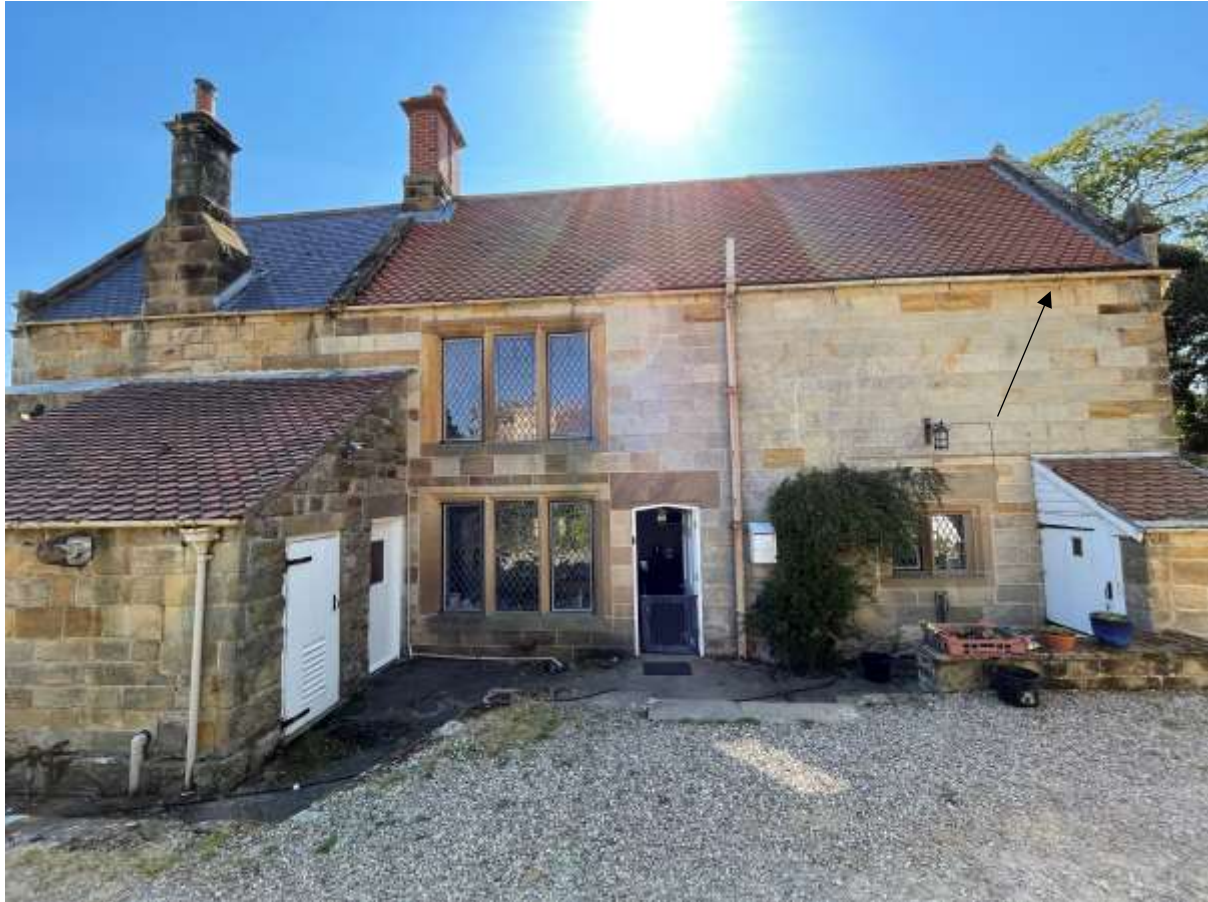
Figure 12 - Northeast Facing Elevation (c.1844) – Guttering arrangement to be renewed. Please note the distance between the roof eaves and the guttering on the RHS of this picture. There is a significant gap between the two which leads to the rainwater shooting over and missing the guttering. This is due to the selected half round profile which does not allow for a significant amount of water within the profile and must be laid at a greater fall, leading to large gaps as the gutter run extends.
