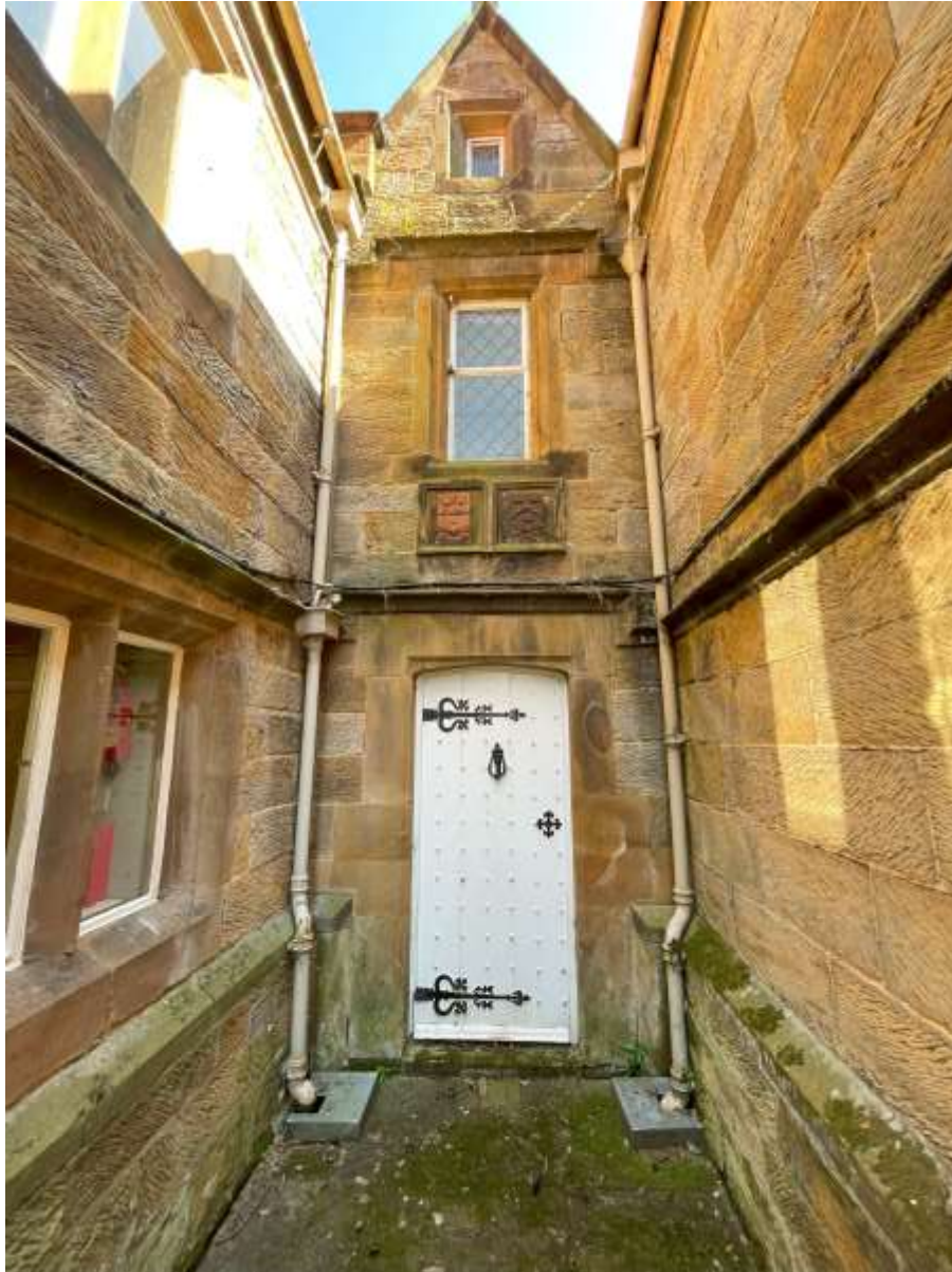
Figure 15 - Northwest elevation of 'Link' building. Downpipes to both sides to be replaced with new. Guttering over to be replaced with new profile. Gulley's and underground drainage to be renewed.
