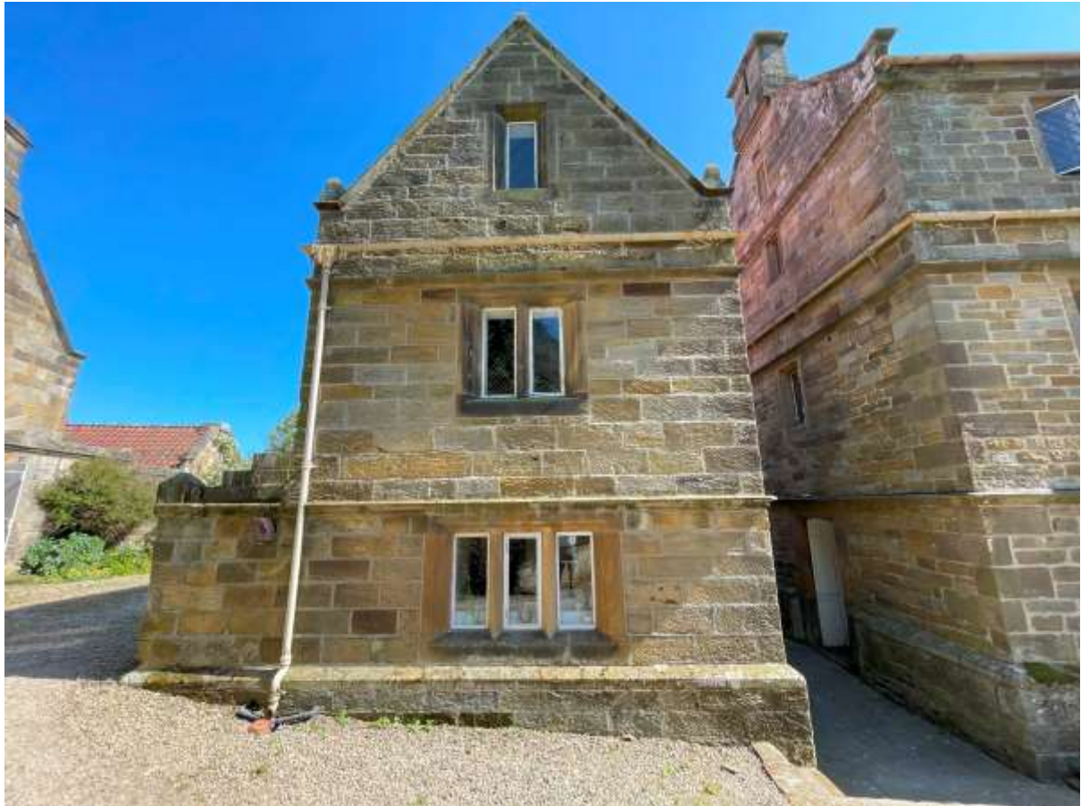
Figure 13 - Northwest Facing Gable (c.1844). Horizontal Gutter at first floor level to be removed. Downpipe to be renewed.
