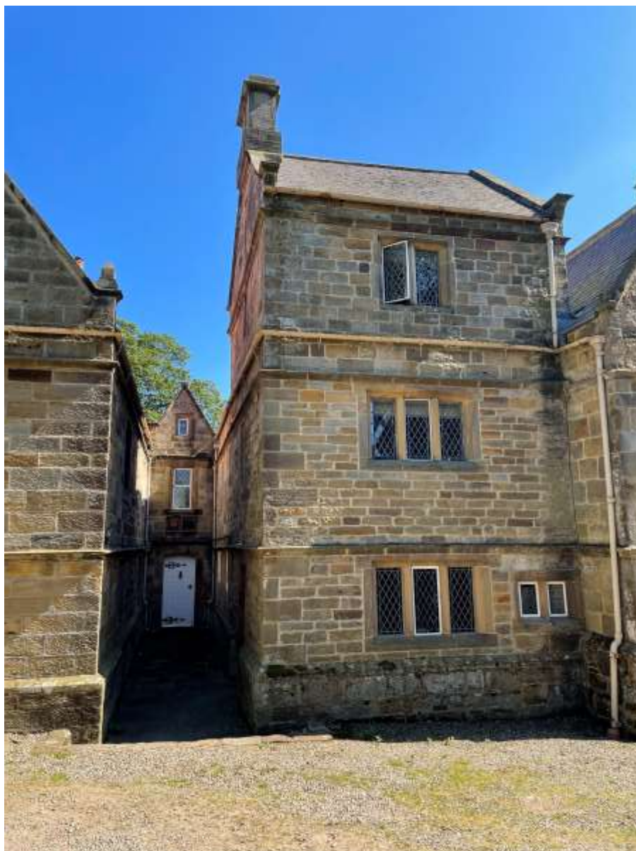
Figure 14 - Northwest Elevation - Storeyed Porch - Horizontal gutter at first floor to be removed. Downpipe and gutter to roof to be renewed. Downpipe to side of 'Original House' to be renewed with new box hopper at top to fix the existing water ingress problems. Please also take note of the roof covering to the storeyed porch. It is proposed this roof is replaced on a like for like basis.
