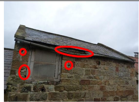
Figure 18: Masonry crevices on rear wall.
