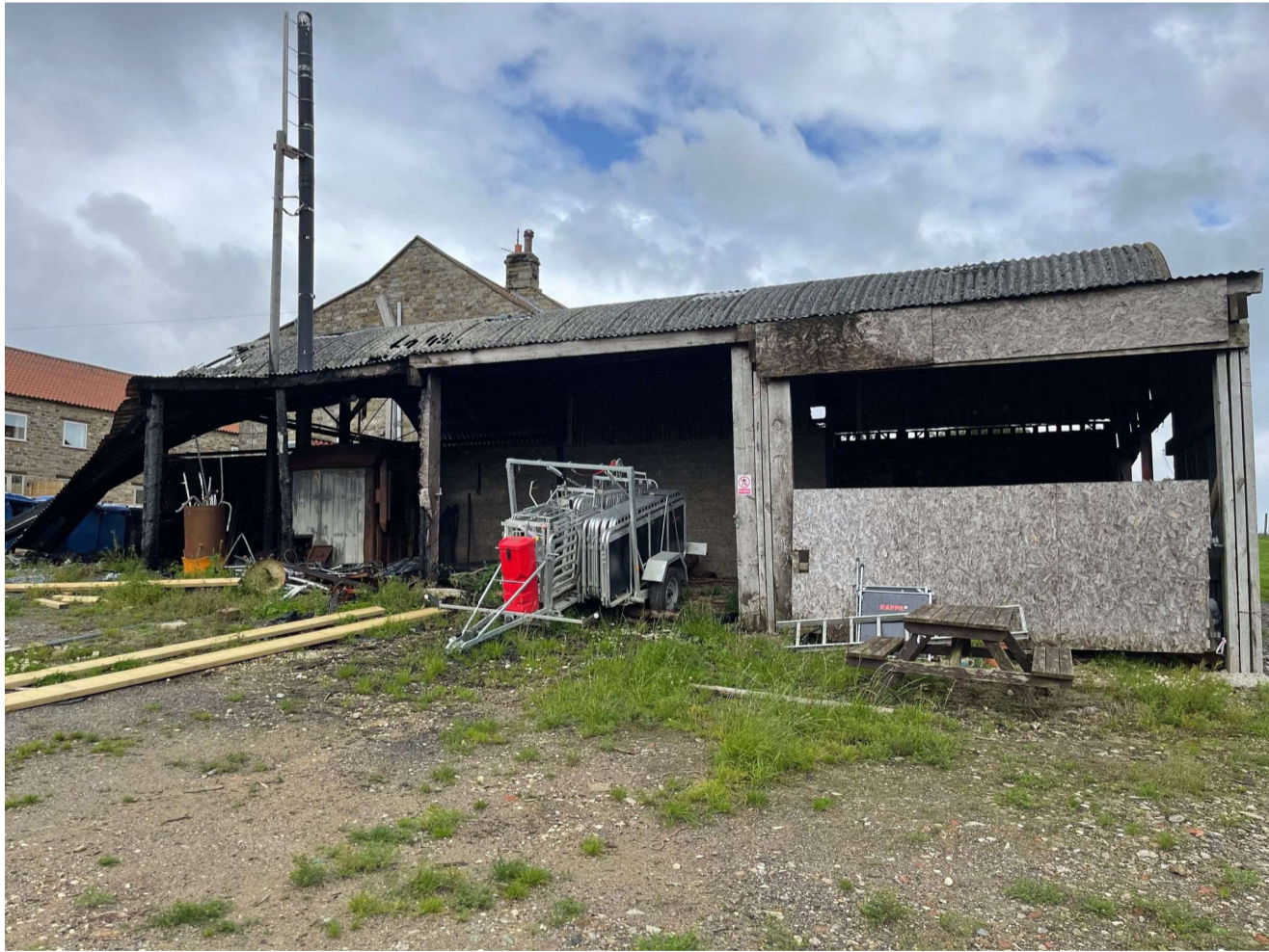
fire damage photo 2
