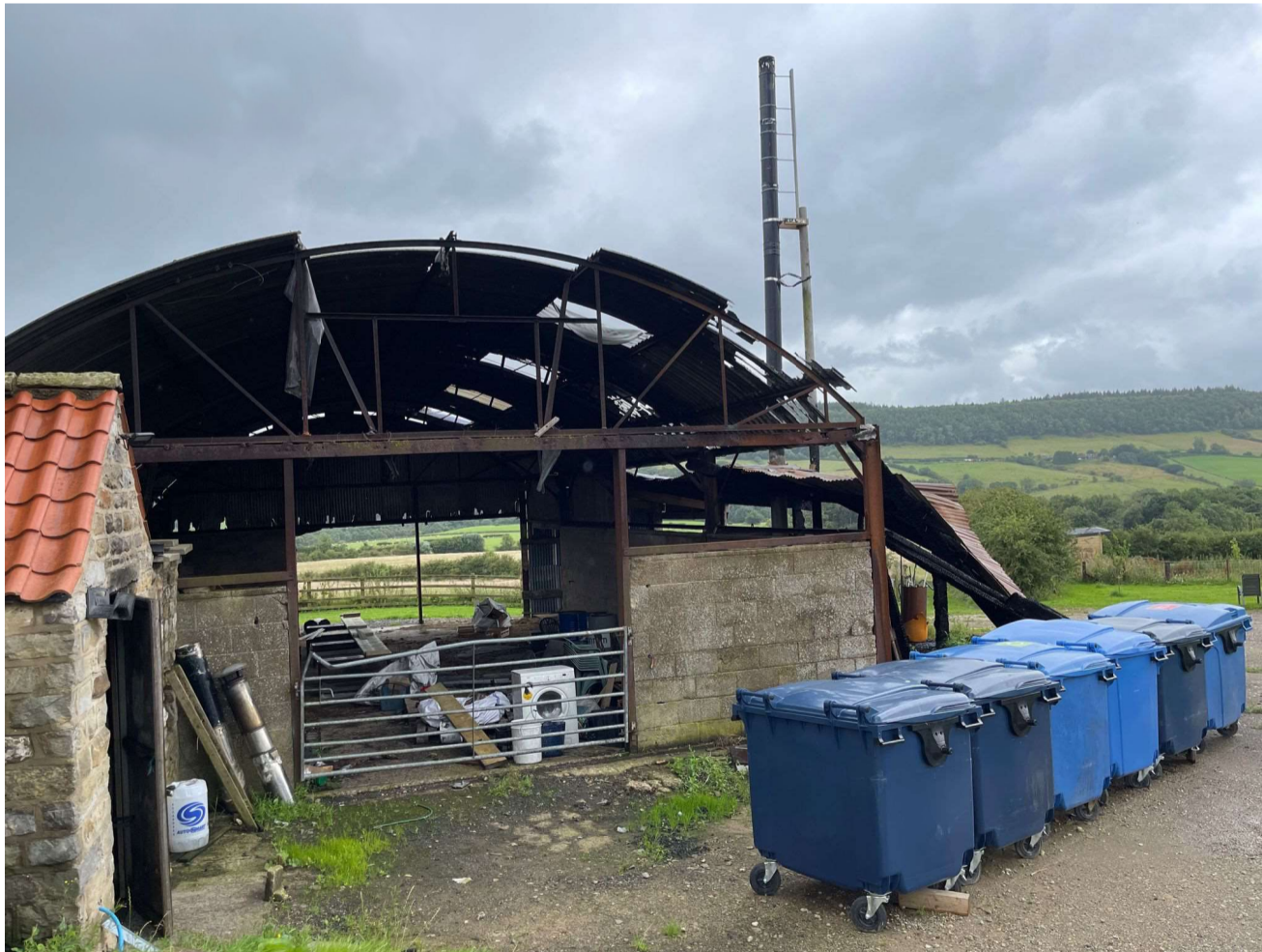
fire damage photo 4
