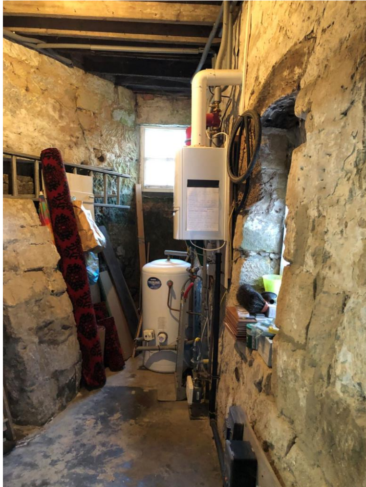
Photo 5 Plumbing and plant in Tapered Room
