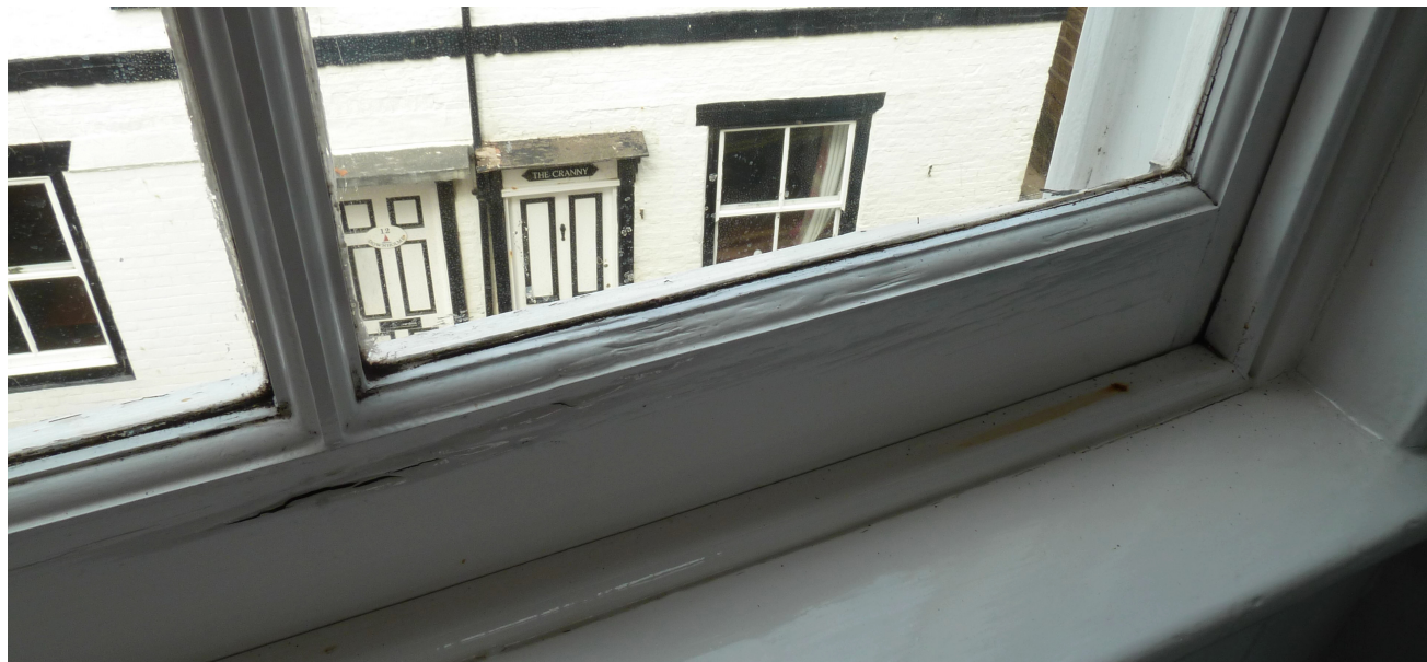
Cracked paint and surface mould indicates general state of decay throughout the frame components internally & externally. Details of the sash and meeting rails as for W2.
